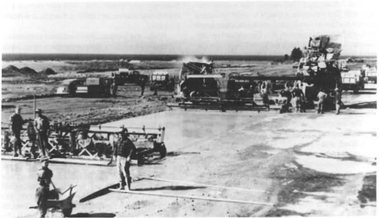
Pavers work both ends of a 25-foot-wide slab on runway at Harmon Field on Newfoundland's west coast.
