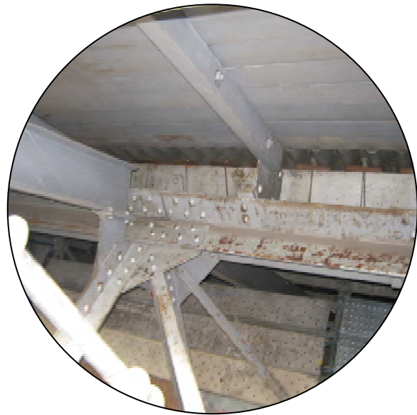
Figure 3-14: Corrosion at Gabled Frame Framing Below Window.
