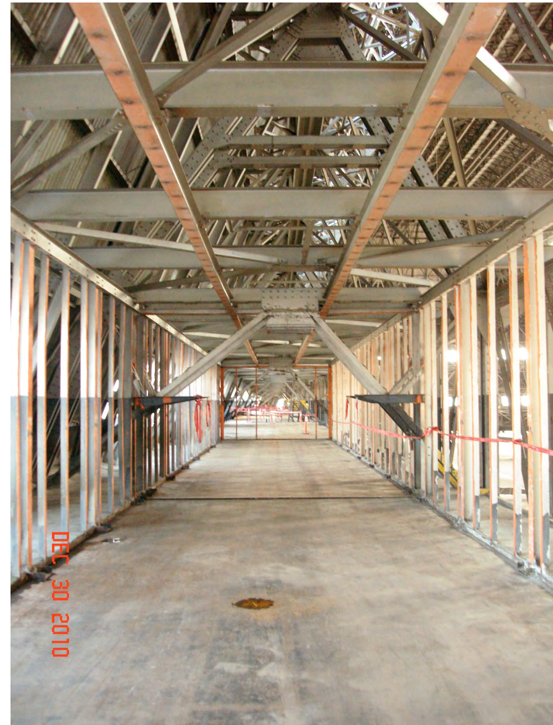
Figure 3-25: Interior Area of Cell Room at Mezzanine
