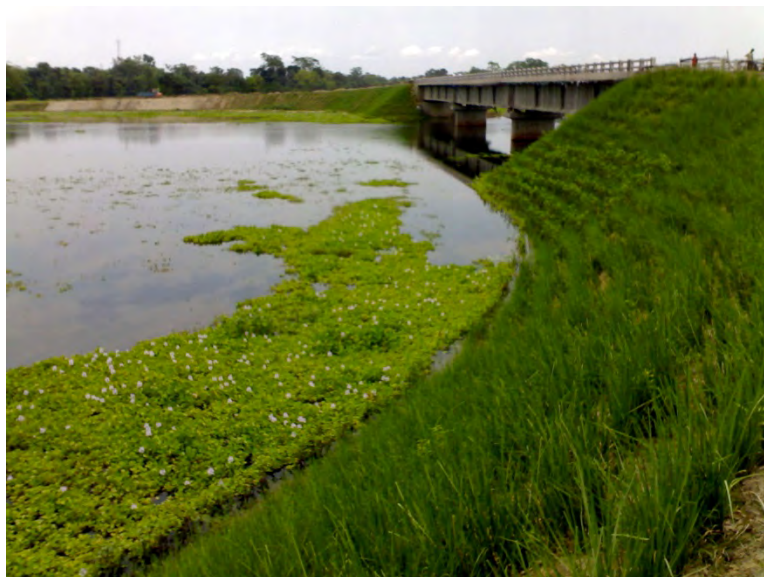
Vetiver has many applications, including slope and streambank stabilization and erosion control (66)
