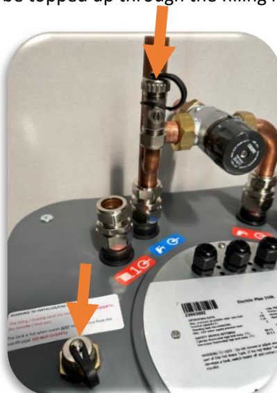
Figure 6 Filling loop disconnected
