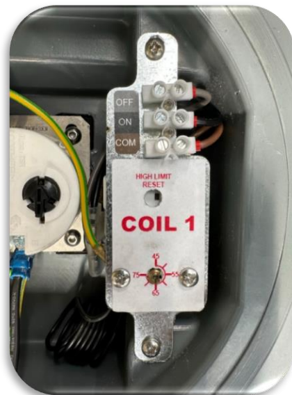
Figure 18 Close up of tank thermostat wiring
