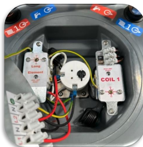
Figure 3 Immersion heater and thermostat compartment
