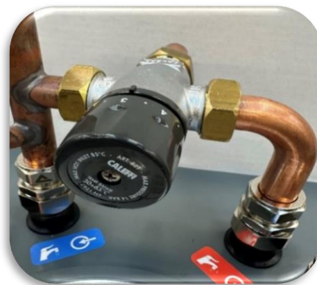
Figure 13 Mixing valve set to position #3
