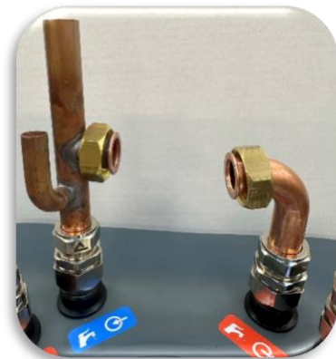
Figure 12 Mixing valve pipe set
