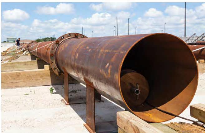
A length of pipeline used for testing by PRCI.
