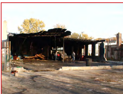
The fire completely gutted Capitol's original building, leaving nothing but a crumbling shell.
