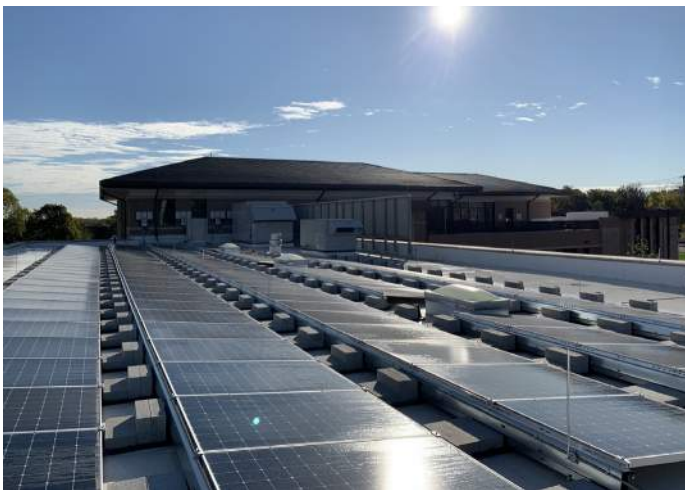
Rooftop photovoltaic panels on the parking canopies helped this project achieve LEED Gold Certification.
