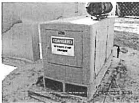
Photo ID #7- Plant #1's generator that serves the system
