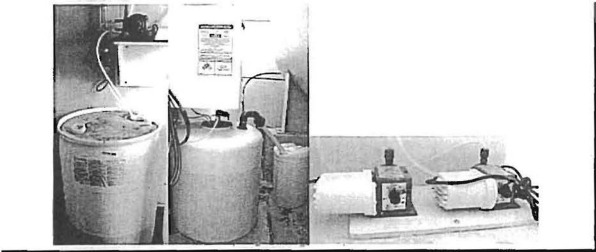
Well 1 - Chloramine Treatment NaClO - Sterner 40 GPD; NH 3 - Chem-Tech 15 GPD x2
