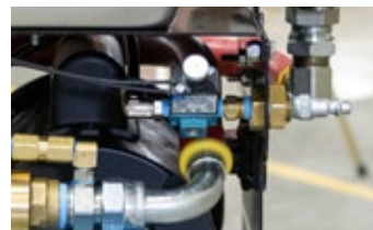
Air purge to additionally agitate during flushing and to clear service lines and cooling system after flushing
