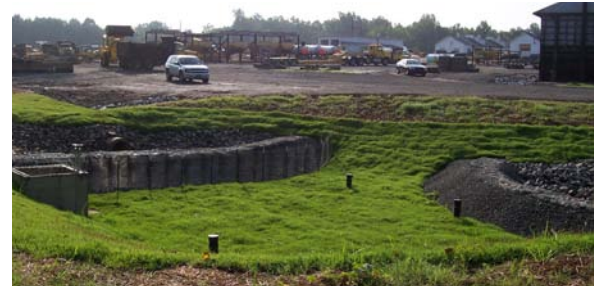
Stormwater control measure implemented at a NCDOT county maintenance yard
