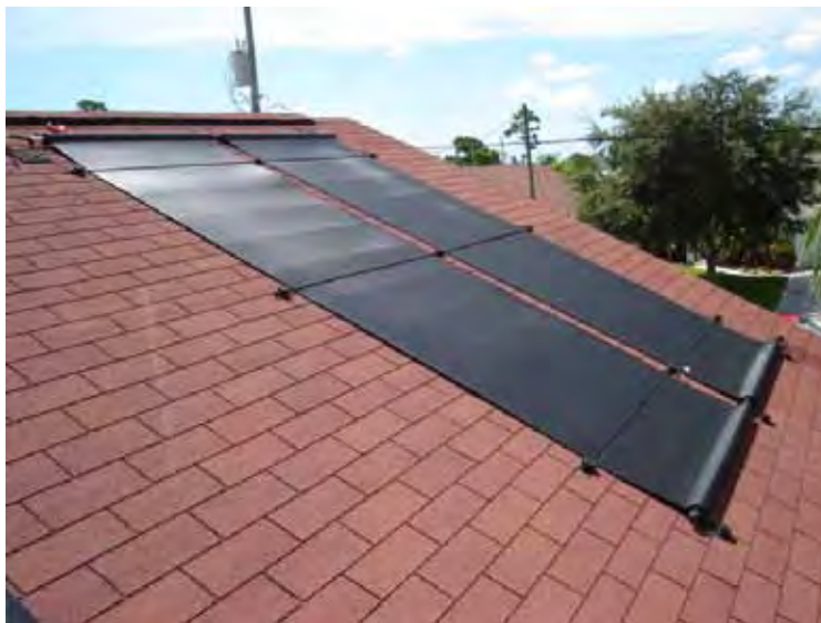
Figure 3.12. An unglazed solar mat-type solar collector made by FAFCO installed on a roof in California.
