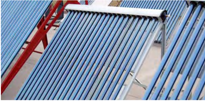
Figure 3.16. SunMaxx evacuated tube solar collectors on the roof of a commercial building.
