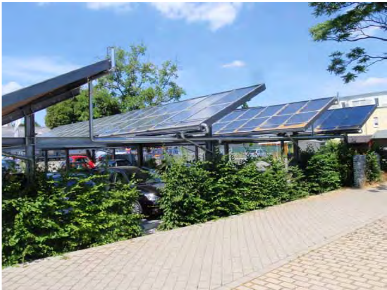
Figure 5.1. Solar hot water collectors place above automobiles where they are parked.
