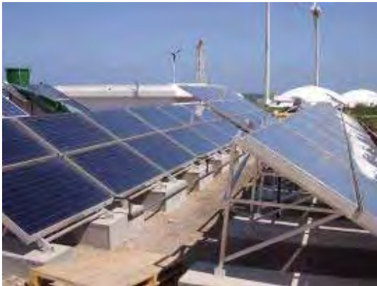
Figure 2.10. Flat plate collectors on mounting construction.
