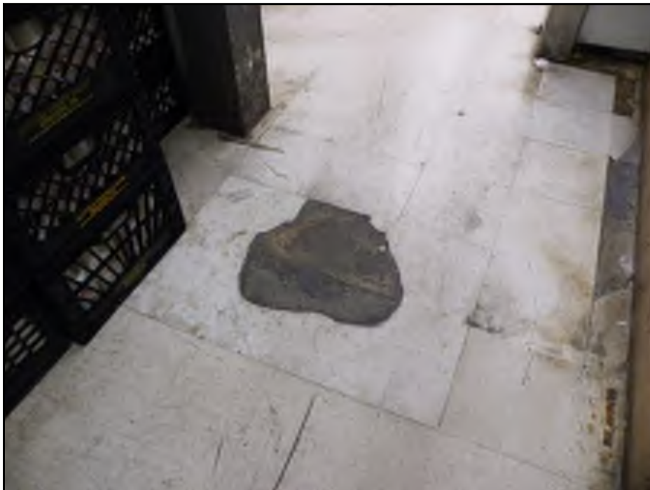
Damaged floor tile
