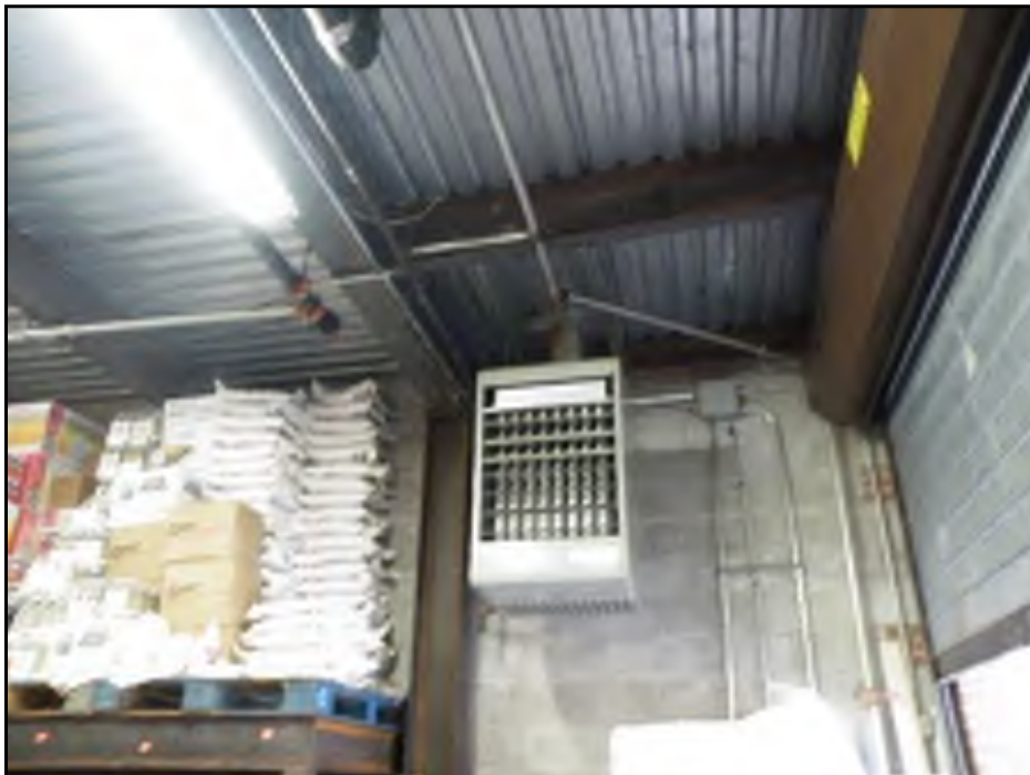
Gas-fired warehouse heater
