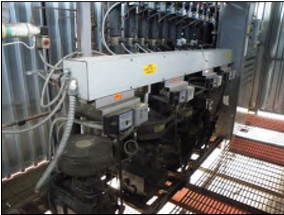
Compressor room (refrigeration)
