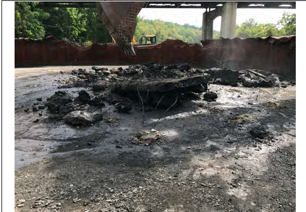
Date: 09/21/2017 Site Name: Troy (Water Street) Site - Area 3 Photographer's Initials: JAJ Description: Photograph #13: Demolition of concrete within Former Tank T-41. Photograph taken facing South.
