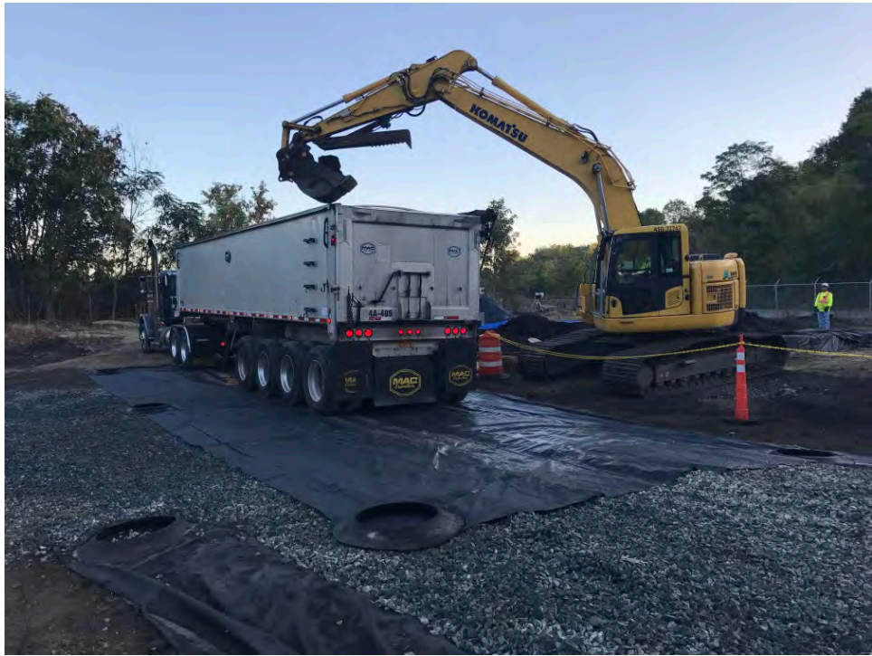
Date: 10/04/2017 Site Name: Troy (Water Street) Site - Area 3 Photographer's Initials: JAJ Description: Photograph #9: Loading of a waste hauler with excavated waste materials staged in the waste staging area. Photograph taken facing Northeast.
