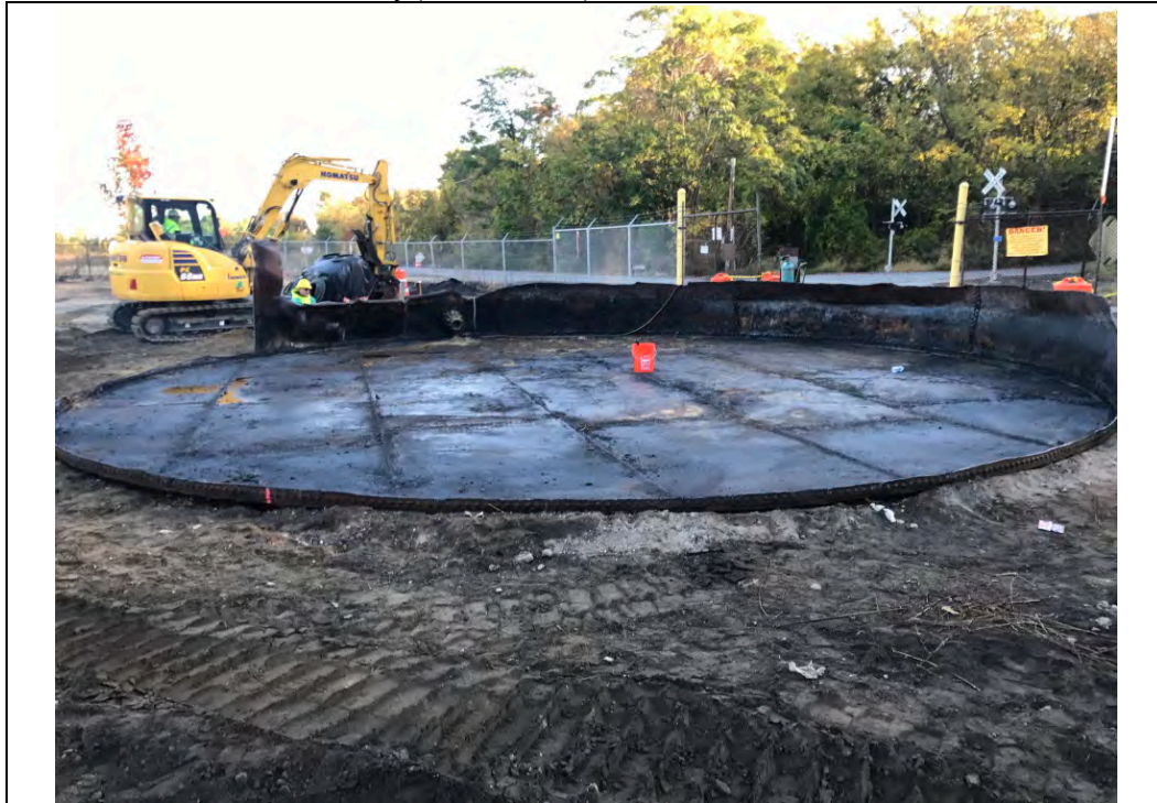
Date: 10/13/2017 Site Name: Troy (Water Street) Site - Area 3 Photographer's Initials: JAJ Description: Photograph #15: Cutting and removal of Former Tank T-41 walls. Photograph taken facing Northeast.
