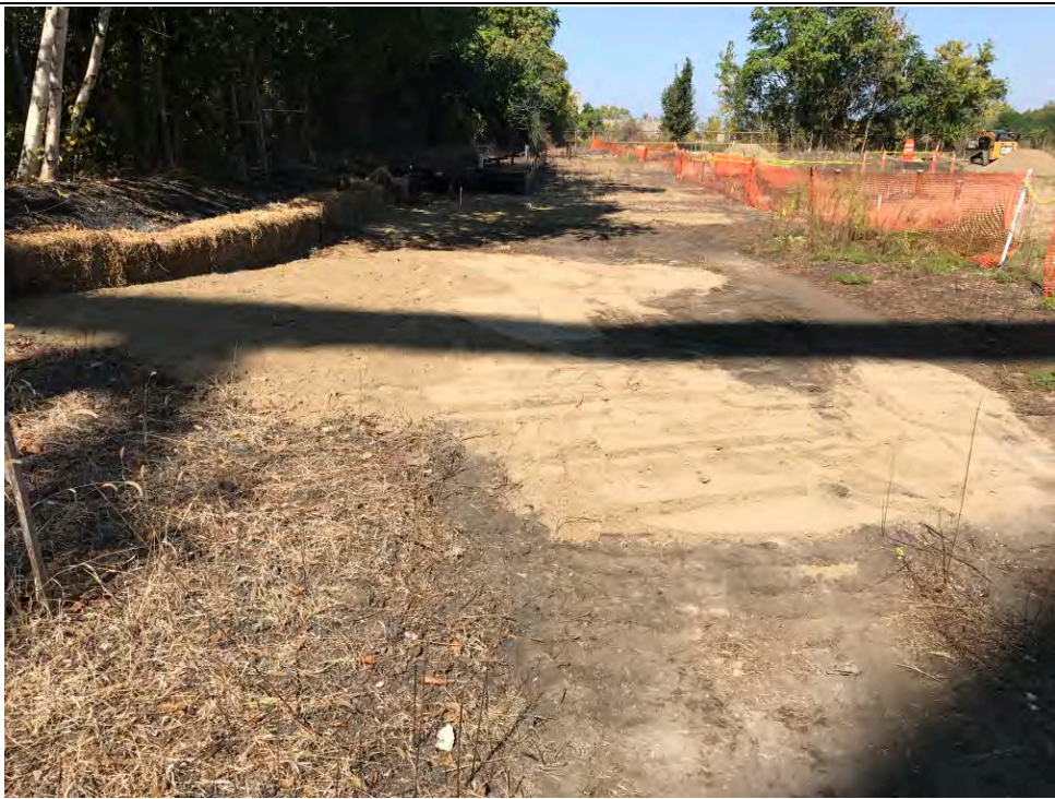
Date: 09/25/2017 Site Name: Troy (Water Street) Site - Area 3 Photographer's Initials: JAJ Description: Photograph #10: Area A-1 backfilled with imported sand and gravel material. Photograph taken facing North.
