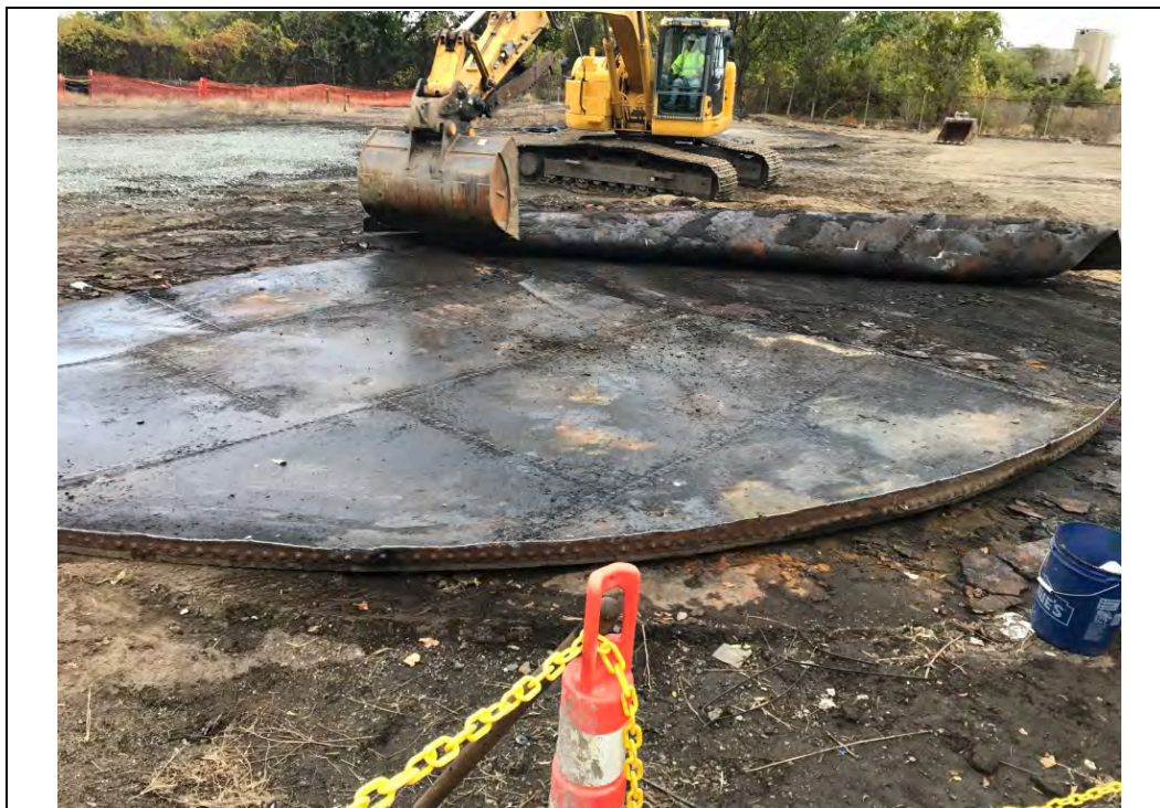
Date: 10/16/2017 Site Name: Troy (Water Street) Site - Area 3 Photographer's Initials: JAJ Description: Photograph #16: Removal of Former Tank T-41 bottom. Photograph taken facing Northwest.
