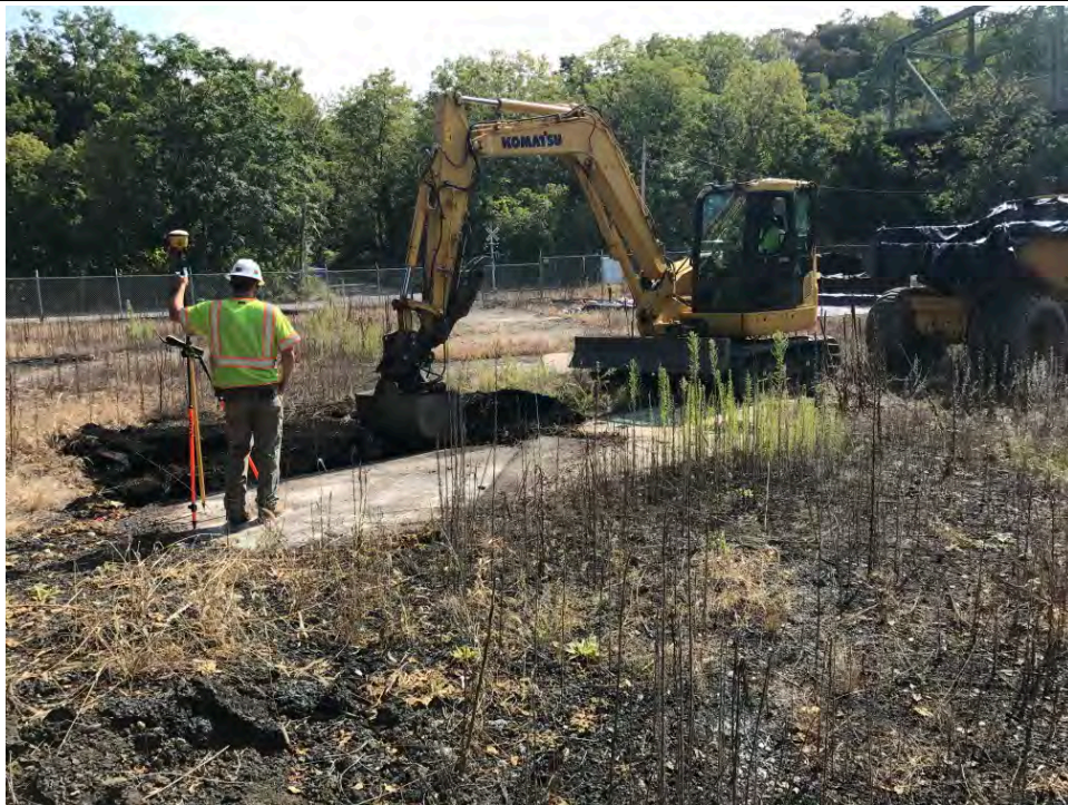
Date: 09/19/2017 Site Name: Troy (Water Street) Site - Area 3 Photographer's Initials: JAJ Description: Photograph #6: Excavation operations at Area A-6. Photograph taken facing East.
