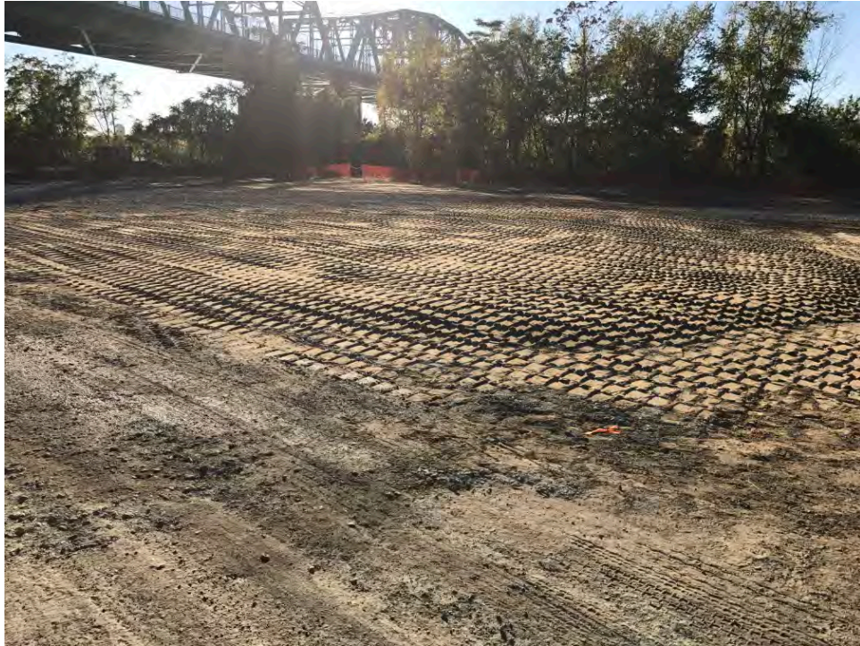
Date: 10/17/2017 Site Name: Troy (Water Street) Site - Area 3 Photographer's Initials: JAJ Description: Photograph #19: Former Tank T-41 area after backfilling with a minimum of eight (8) inches of imported sand and gravel material. Photograph taken facing Southwest.
