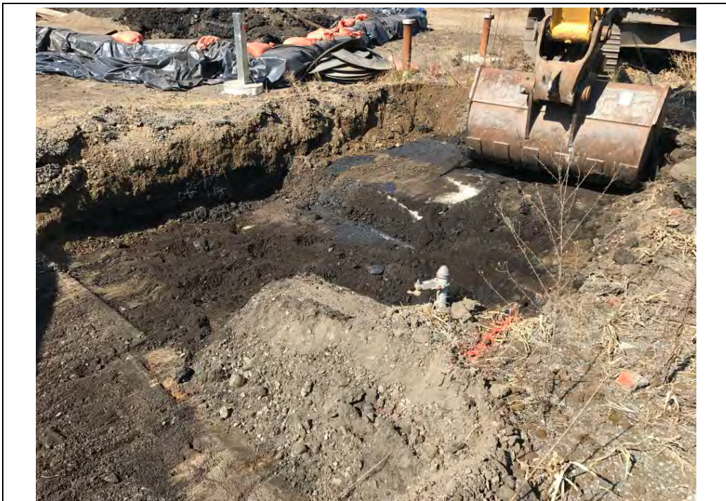
Date: 09/25/2017 Site Name: Troy (Water Street) Site - Area 3 Photographer's Initials: JAJ Description: Photograph #8: Excavation operations at Area B-1. Photograph taken facing Northeast.
