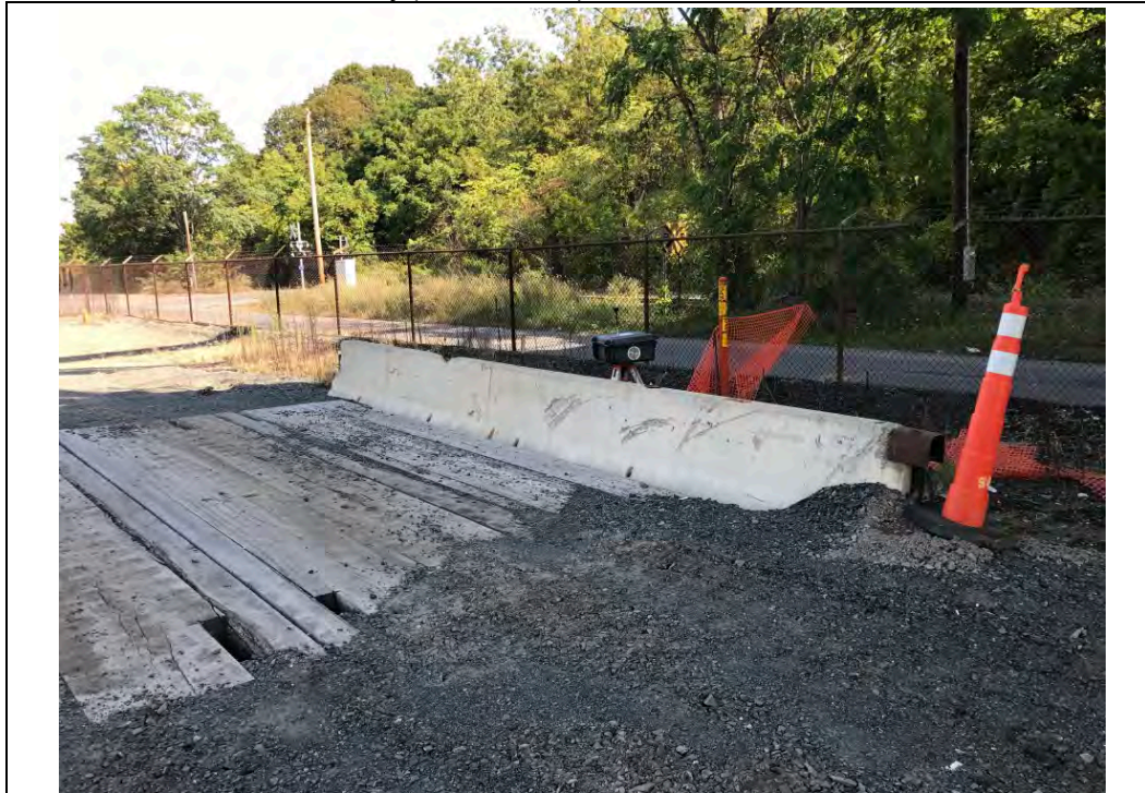
Date: 09/19/2017 Site Name: Troy (Water Street) Site - Area 3 Photographer's Initials: JAJ Description: Photograph #1: Air bridge installed over existing gas main. Photograph taken facing Northeast.
