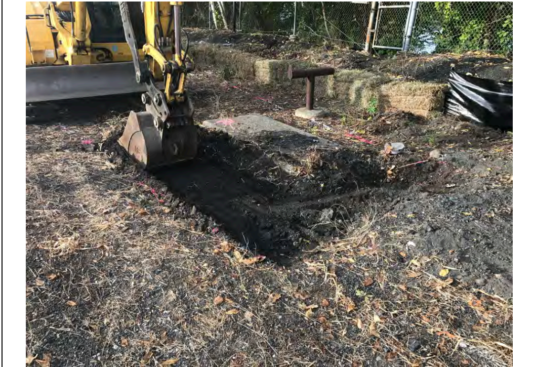
Date: 09/20/2017 Site Name: Troy (Water Street) Site - Area 3 Photographer's Initials: JAJ Description: Photograph #7: Excavation operations at Area A-2. Photograph taken facing Southwest.
