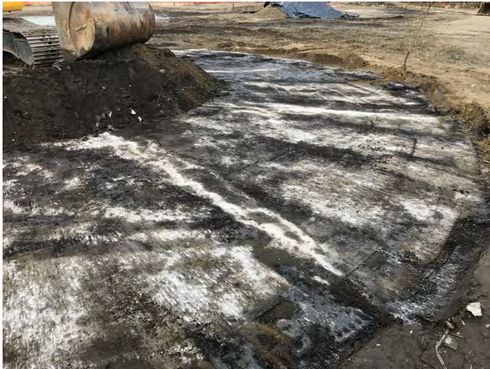
Date: 10/16/2017 Site Name: Troy (Water Street) Site - Area 3 Photographer's Initials: JAJ Description: Photograph #17: Excavation of tar-impacted soils below the Former Tank T-41 steel structure.
