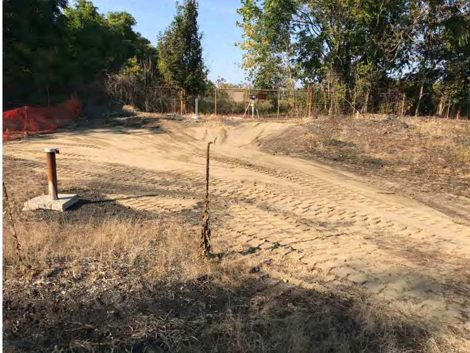
Date: 09/25/2017 Site Name: Troy (Water Street) Site - Area 3 Photographer's Initials: JAJ Description: Photograph #11: Area A-5 backfilled with imported sand and gravel material. Photograph taken facing North.
