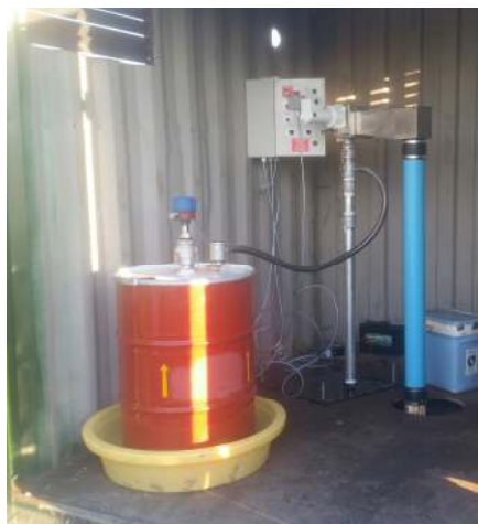
NAPL recovery NET System in operation
