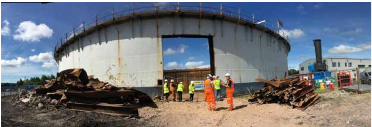
Window to a future, photograph courtesy of National Grid
