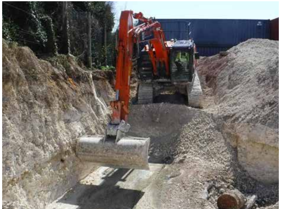
Exposure of the concrete cap on a burial pit
