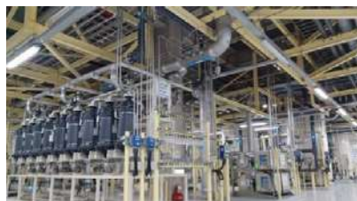
Energy recovery from UPW system for reuse
