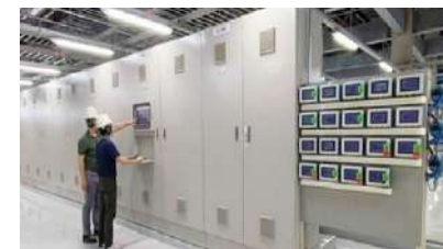
Energy-saving system for the chilled water system
