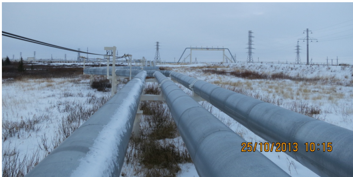
Figure 1. Part of the aboveground pipeline with a diameter of 220 mm
