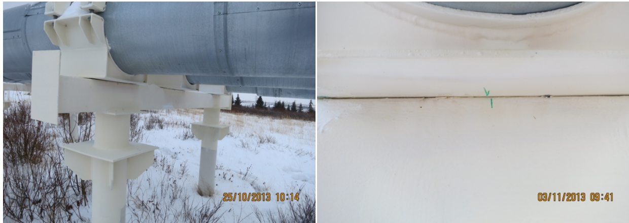
Figure 5. Displacement of the aboveground pipeline at the support #409.
