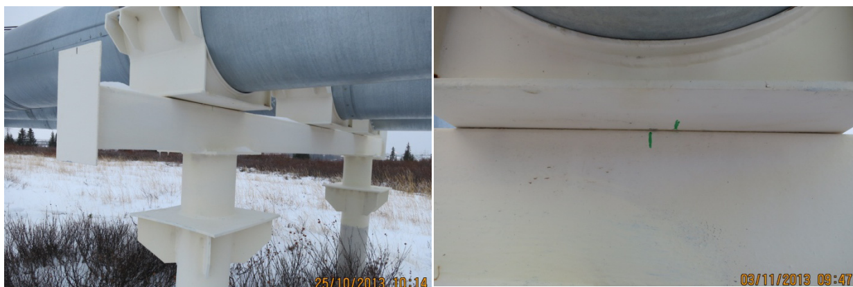
Figure 4. Displacement of the aboveground pipeline at the support #407
