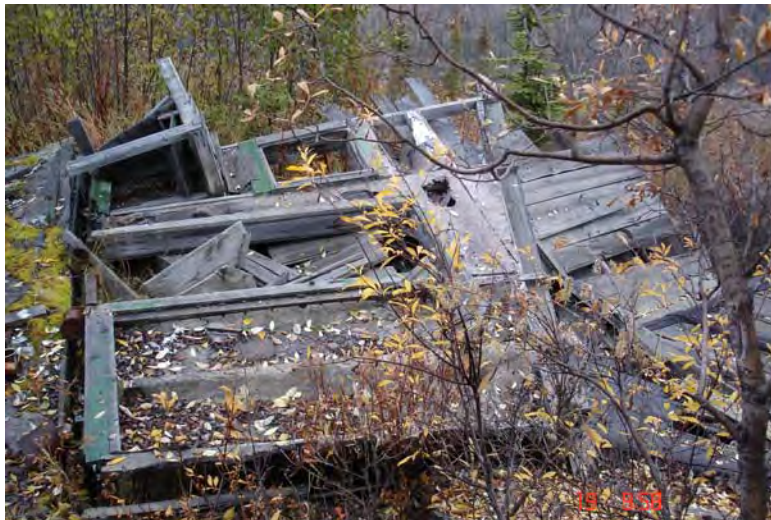
Photo 22.15_Shaft at 100 Level with collapsed structure
