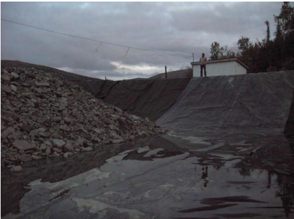
FIGURE 14. SHOWS LINER AND INITIAL LOADING OF COARSE STREAMBED (PLACER) ROCK INTO THE LINED REACTOR.
