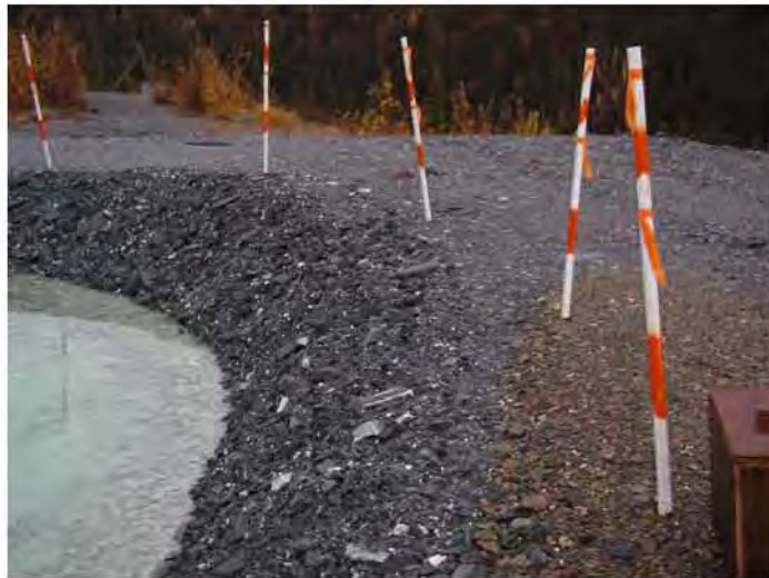
Photo 22.7_Bellekeno tension cracks on upstream crest
