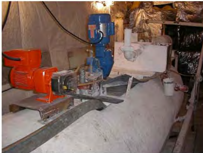
Photo 22.2_Bellekeno lime tank and pumps
