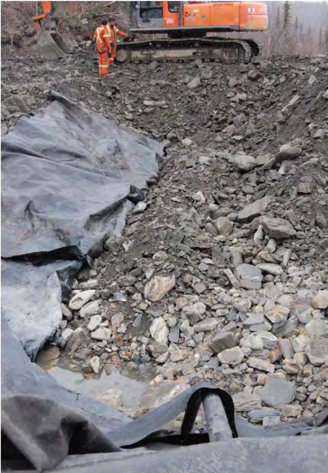
FIGURE 15. PLACEMENT OF ROCK IN REACTOR. NOTE LINER BAFFLE ON THE LEFT, DRAINPIPE IN THE CENTER BOTTOM.
