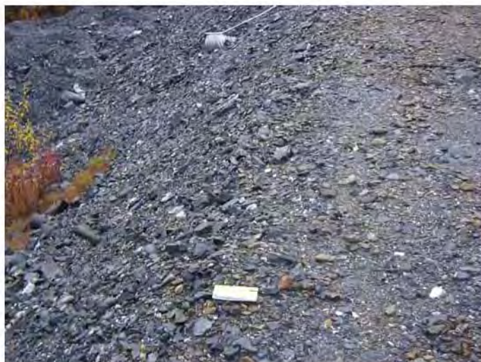
Photo 22.8_Bellekeno tension cracks on downstream crest
