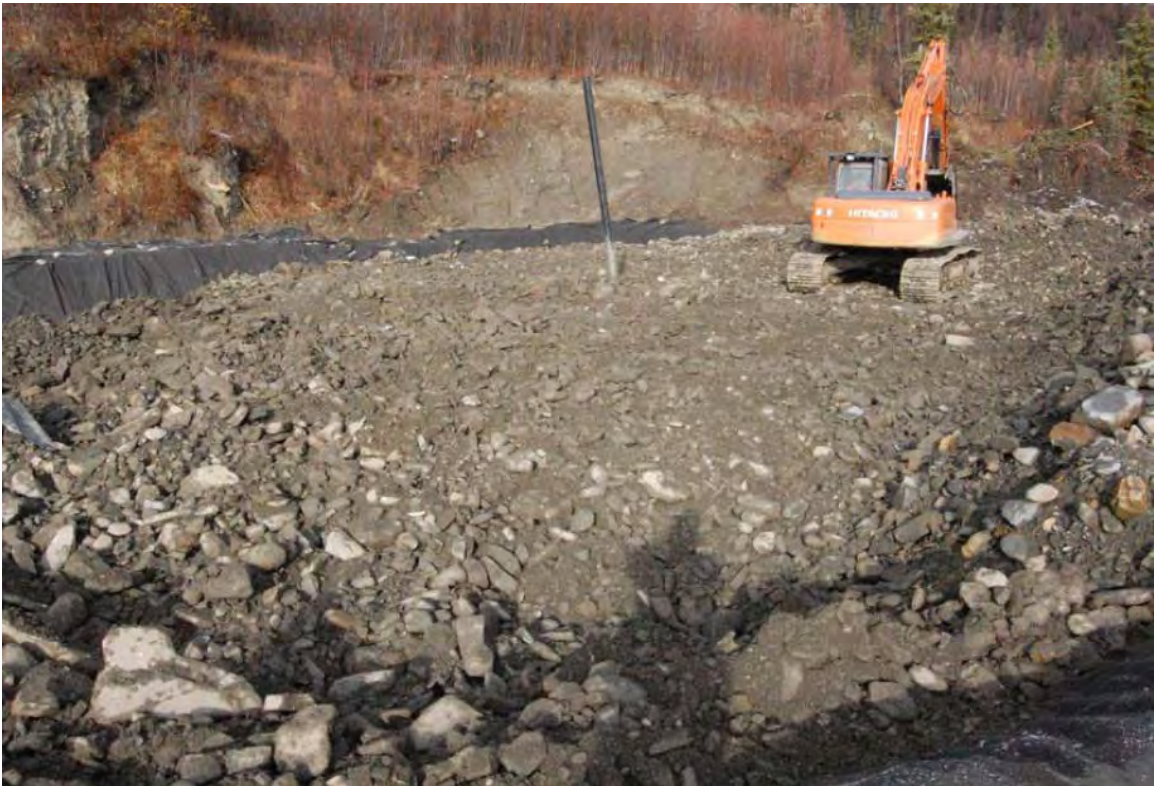
FIGURE 16. PLACEMENT OF ROCK WITHIN BIOREACTOR. NOTE SAMPLING STANDPIPE IN CENTER OF PICTURE.
