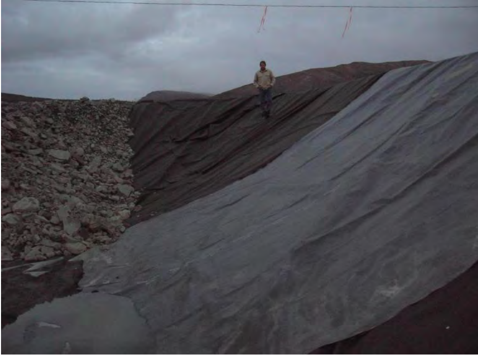
FIGURE 13. SHOWS LINER AND INITIAL LOADING OF COARSE STREAMBED (PLACER) ROCK INTO THE LINED REACTOR.
