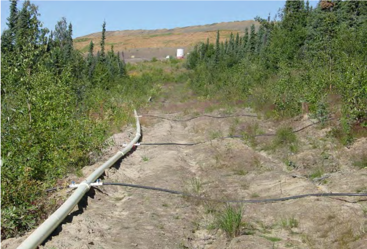
Figure 1. Alexco installed land application system at Brewery Creek Mine
