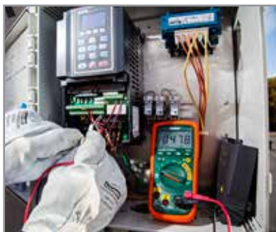
Low Pass Filter (LPF) ensures accurate AC Voltage measurements on a variable frequency drive.
