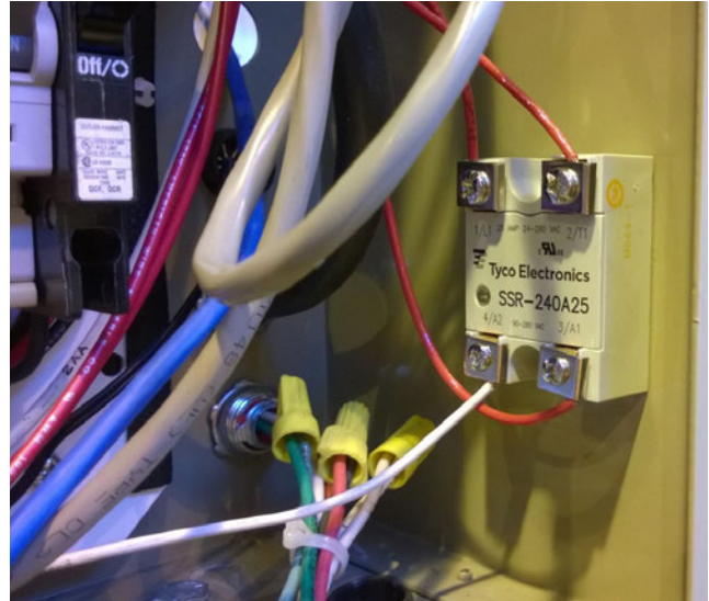
Figure 33. Installed solid state relay
