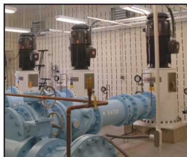
Interior of pump station
