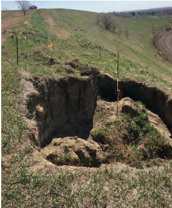
Large Sink Hole on Crest
