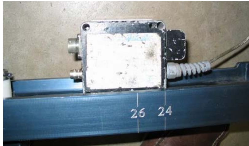
Figure 10.19 Placement of Shunt Resistor Box
