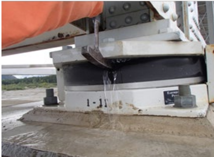
Figure 1.3. Water contamination in Robertson River Bridge (Alaska DOT&PF, 2019).
