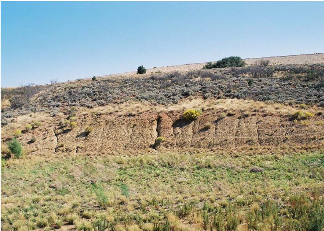
MNT 9/2005. PL-6. Baseline photo taken in 2004 from center of Sediment Pond A dam documenting erosion on south side of pond.
