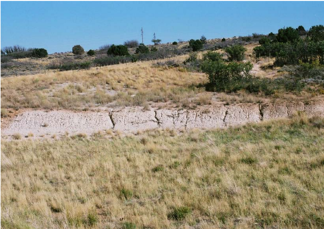
MNT 9/2005. PL-4. Baseline photo taken in 2004 from center of Sediment Pond B dam documenting erosion on south side of pond.
