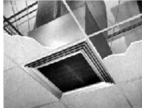
COMMERCIAL "T" BAR CEILING
