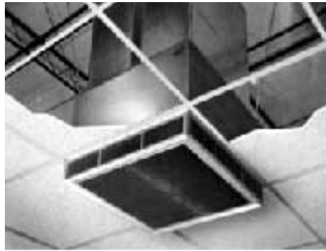
COMMERCIAL "T" BAR CEILING
