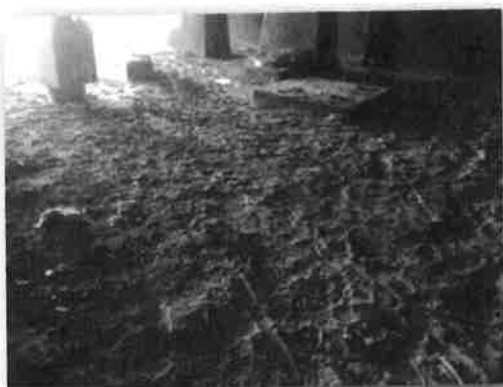
Loose Soil in Crawl Space (Bulk PCB Remediation Waste)
