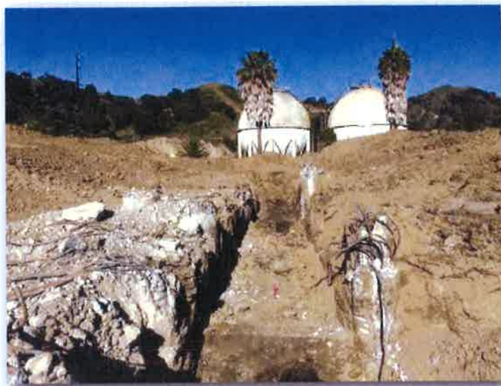
Round 2 Sampling Trench (Sample IJ17.5 in Foreground; FNDL PIPE Visible in Background)
