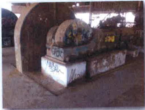
Oil Staining on Compressor No. 1 at Building Floor Deck Level (part of original oily material cleanup)
