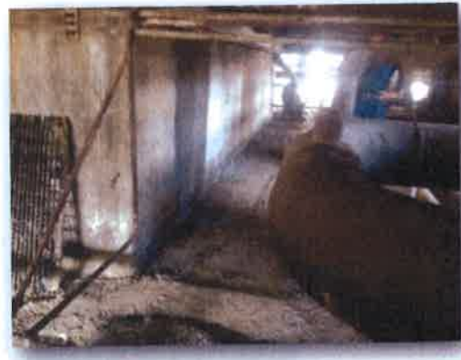
Oil Staining on Compressor No. 1 Foundation in Crawl Space Below (part of original oily material cleanup)
