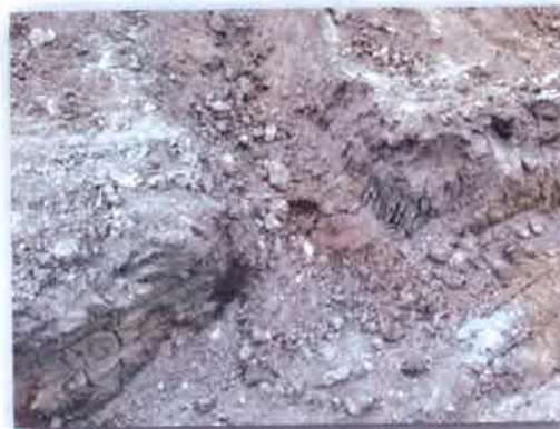
FNDL PIPE Termination at Wye (Vicinity of IJ13.5)
