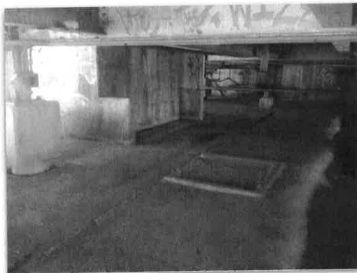
Typical Concrete Filled Sump
