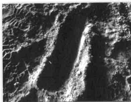
Detail of Loose Soil Note Concrete Slab Below
