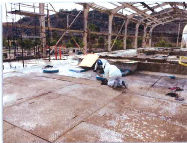
Decontamination of Gross Residues in Floor Deck Area During Interim Cleanup (note painted steel diamond plate floor coverings)
