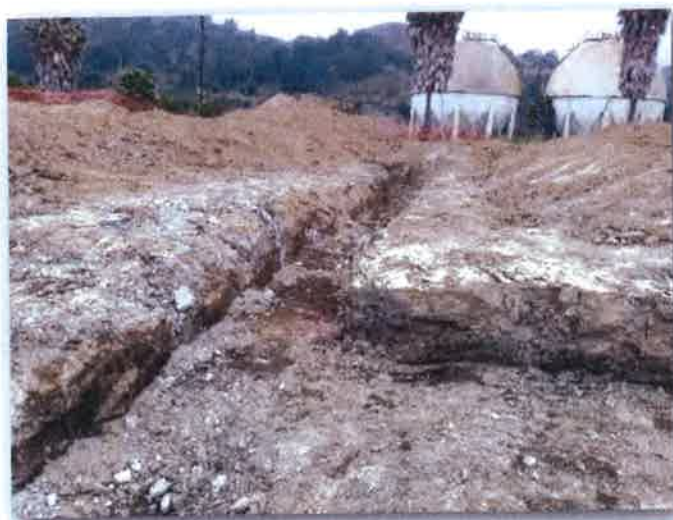
Staining Prior to Round 4 Excavation ( FNDL PIPE is below staining level in Row IJ trench)
