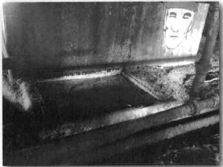
Gross Residues in CrawlSpace (Note Concrete-Filled Sump)
