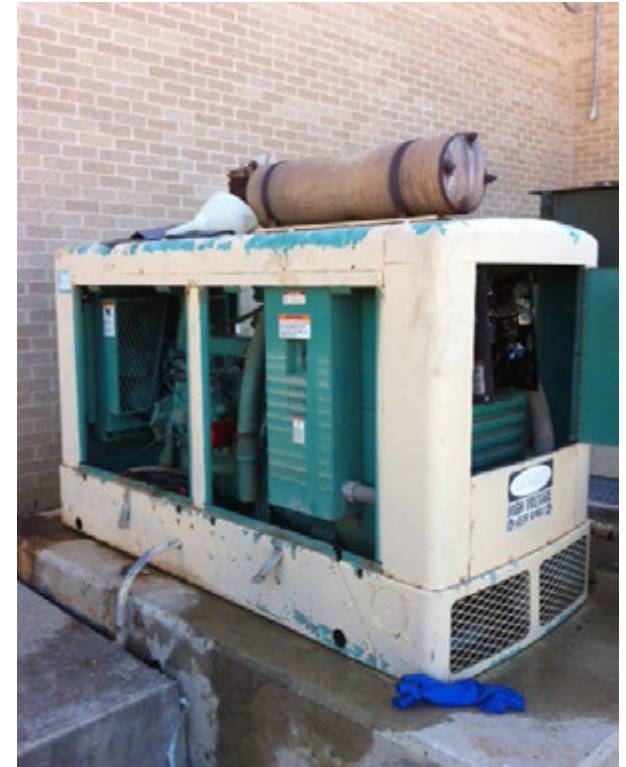
STUDENT RECREATION CENTER GENERATOR
