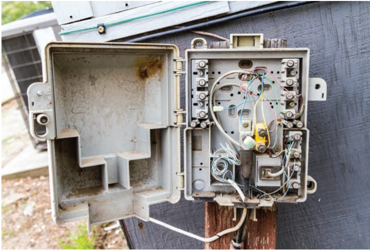
Figure 11-6 A Telephone System Demarcation Point
