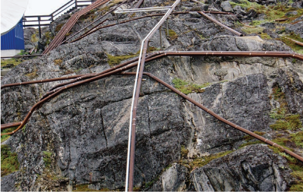
Figure 12-2 Cables Attached to Rock in Nuuk, Greenland
