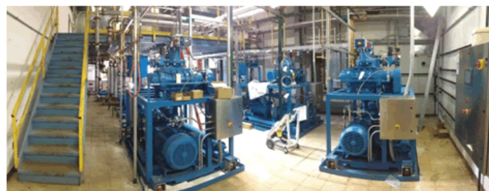
Figure 4. Liquid Helium Facility
