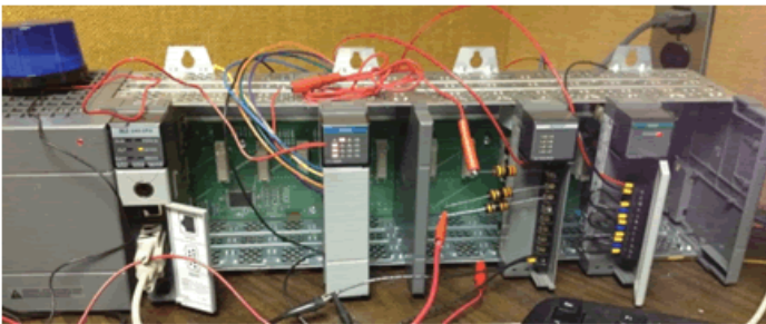
Figure 1. PLC processor with I/O modules
