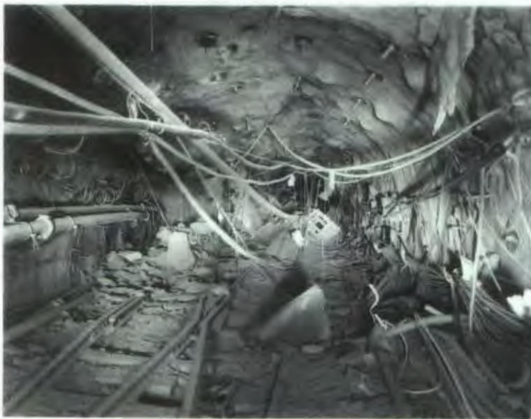
Figure 3 Photo showing damage at the intersection of the North Access drift to the Fast alcove and the U12n.23 Access drift. Caving in the North Access drift (left background) and floor heave are evident. View is to the WP from CS 4+60 of the U12n.23 Access drift (see Figure 2). Photo by Johnson Controls.
