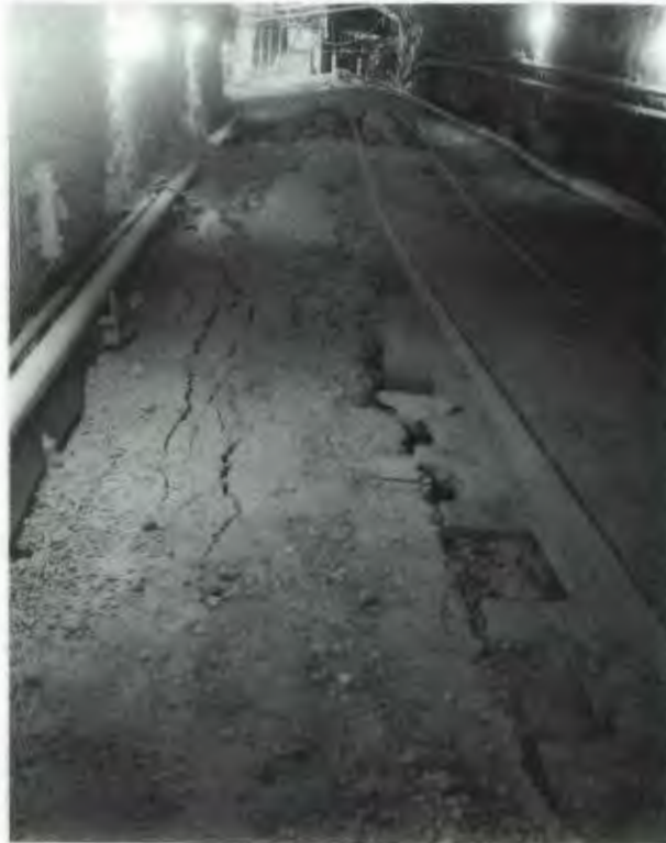
Figure 4 Photo showing area of maximum floor heave and tilt in the N-Extension South drift. Possible pressure ridge extends from left foreground to rail spur in the background. View is toward the portal from approximately CS 55+60 (see Figure 2). Photo by Johnson Controls.
