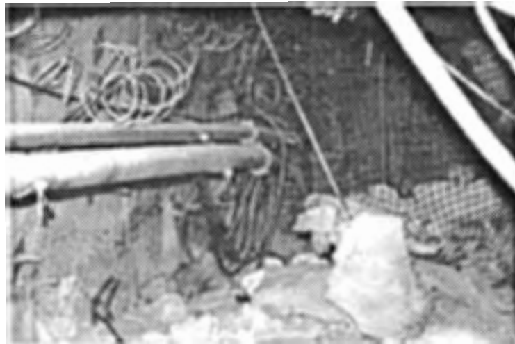
Figure 14. The pressure lines may have been pinched off by falling rock.
