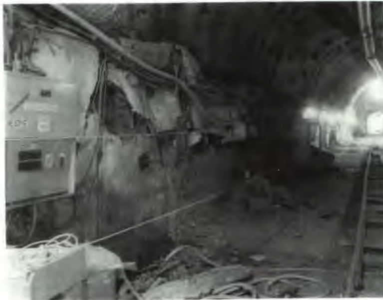
Figure 5 Photo showing slabbing along the left rib of the North Experiment alcove 1.2 m above the invert. View is from intersection of the N-Extension North drift and the N-S Connecting drift (see Figure 2). Photo by Johnson Controls.
