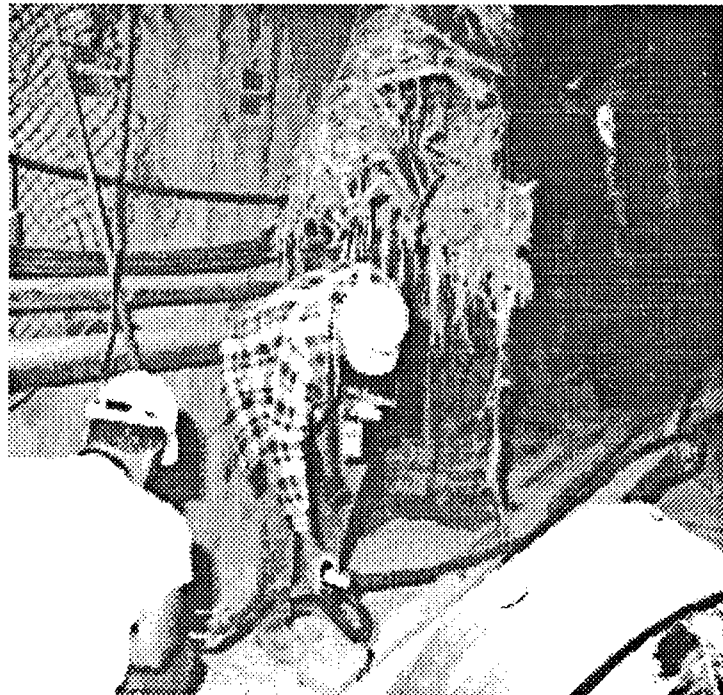
Figure 16. Damage to tunnel and ducting in vicinity of the experiments.
