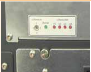
Fan failure display/four speed levels
