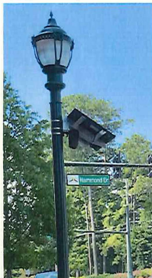
Solar & Existing Pole
