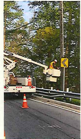
Electric & Existing Pole
