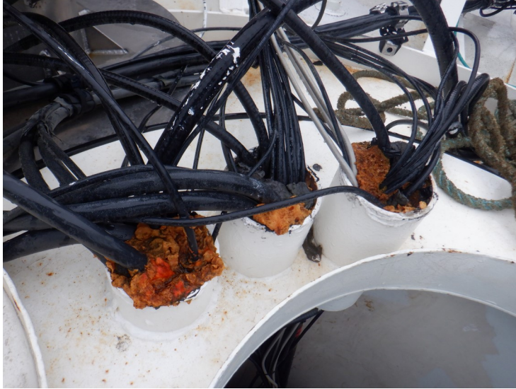
28) The spray foam insulation in the cable routing penetration pipes through the access tube cover plate is deteriorating.
