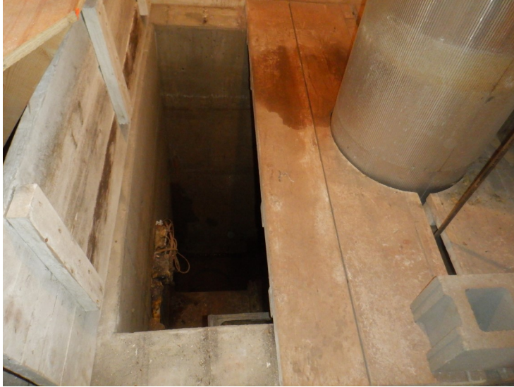
79) The wooden cover over the pit in the basebell is in good condition.
