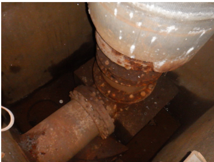
81) The coating on the pit piping is in poor condition.
