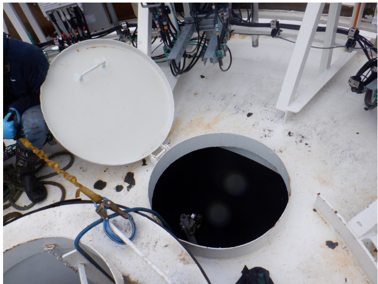
26) There is no gasket on the wet interior roof hatch.
