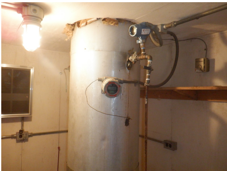
39) The sample tap on the fill/draw pipe in the basebell is in good condition.
