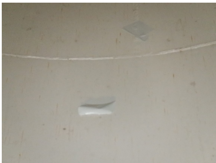
45) There are a few coating failures in the dry riser.
