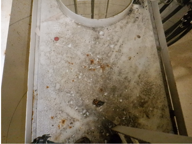
52) There are a few coating failures on the top platform.
