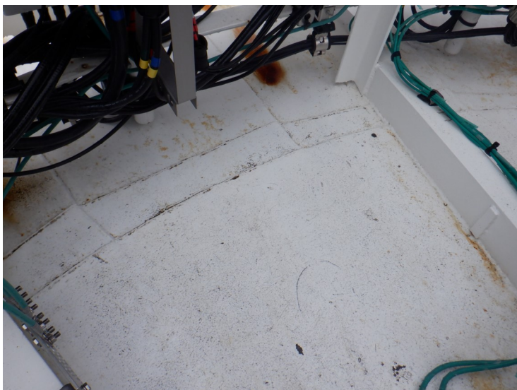
21) There are a few coating failures on the roof. The coating is in good condition overall.
