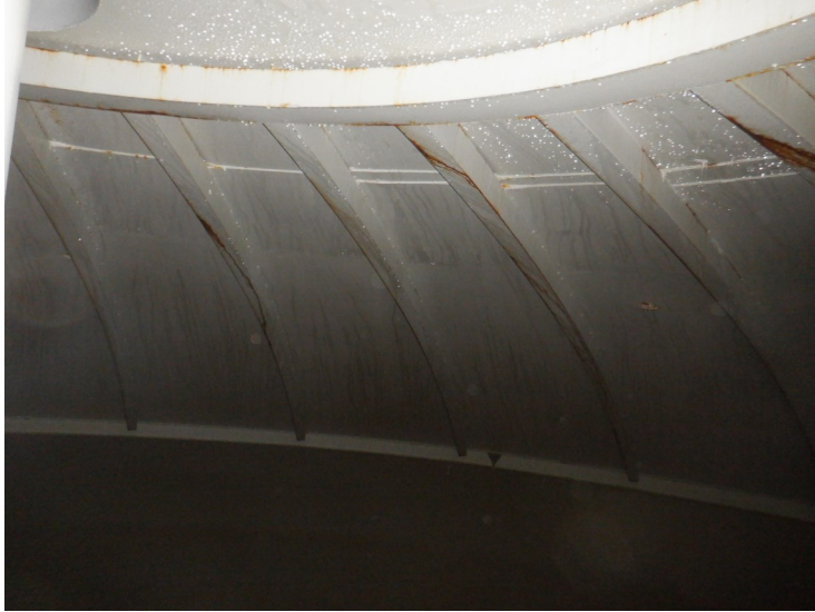
64) There is minor corrosion on the roof stiffeners in the wet interior.
