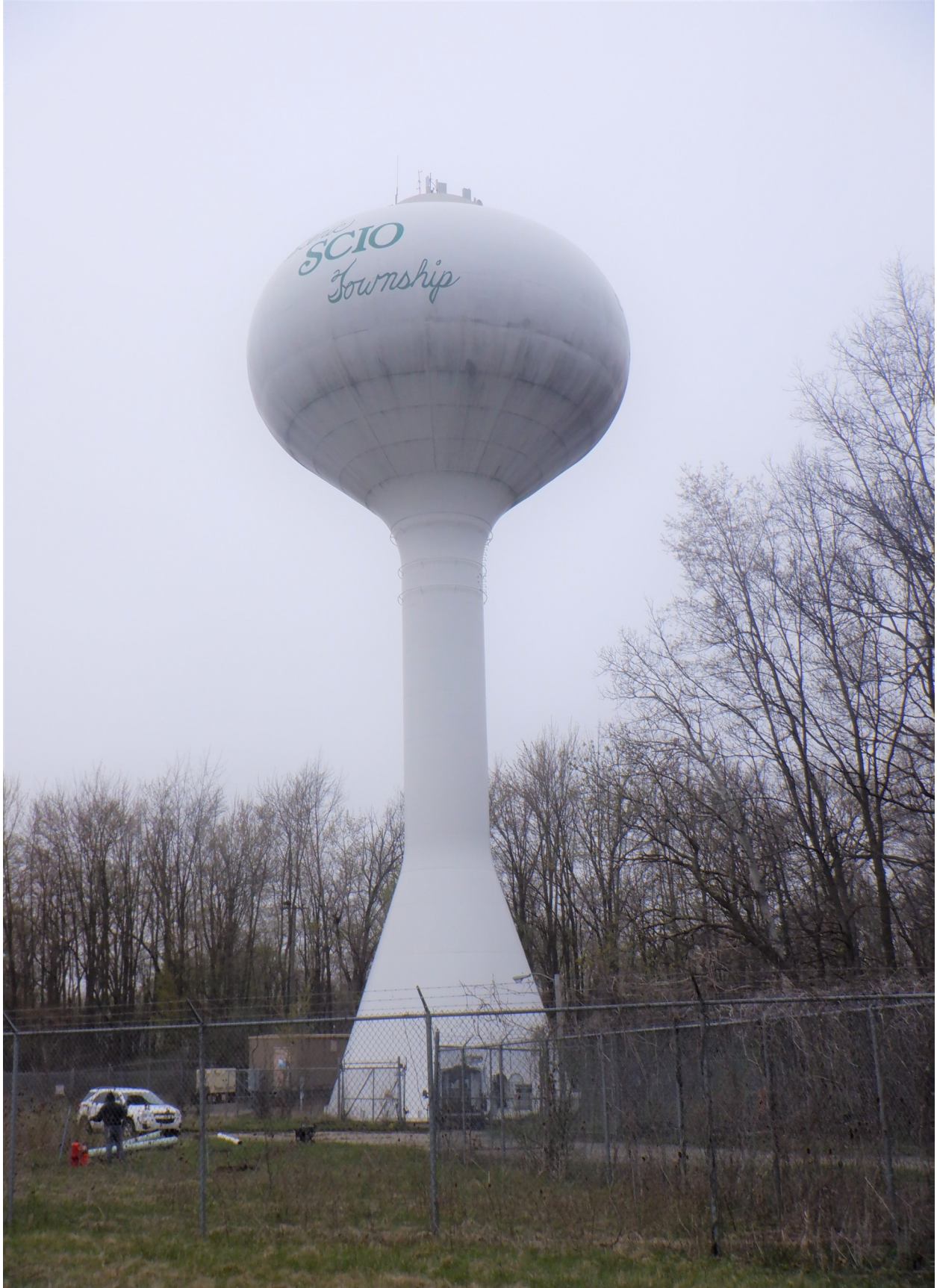
1,000,000 gallon spheroid elevated water storage tank located in Ann Arbor, Michigan and owned by Scio Township.
