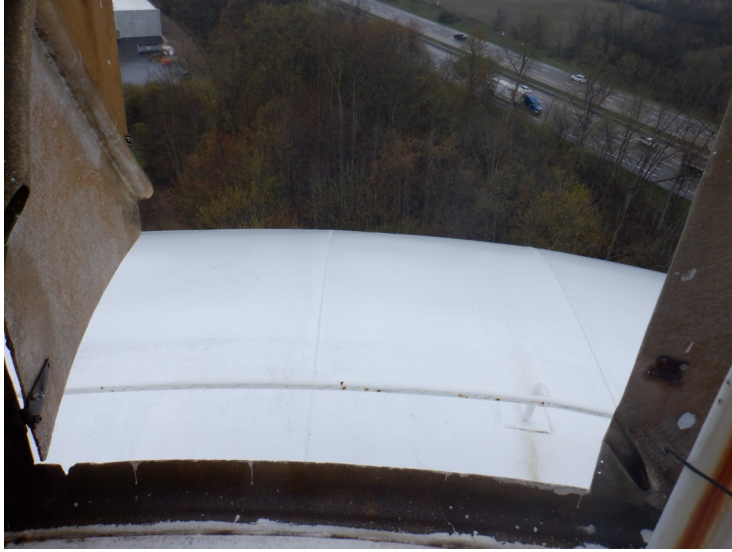
22) Roof top fiberglass shroud hinged door does not stay closed. Needs attention.
