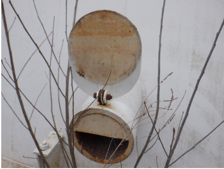
7) There is no screen at the overflow pipe discharge.
