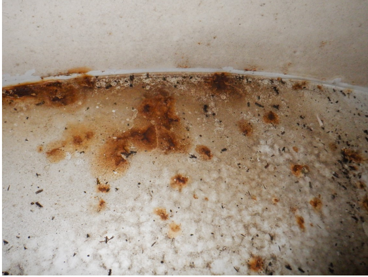
43) The coating on the condensate platform is in fair condition with a few failures.
