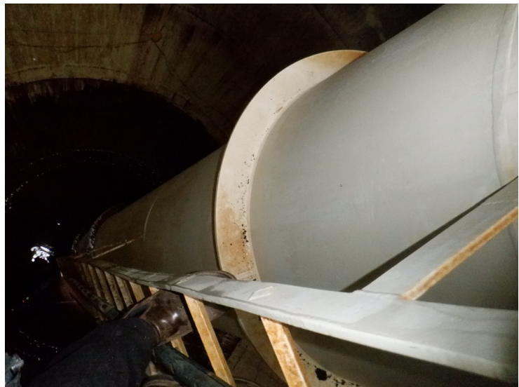
74) The access tube coating in the wet interior is in good condition overall.
