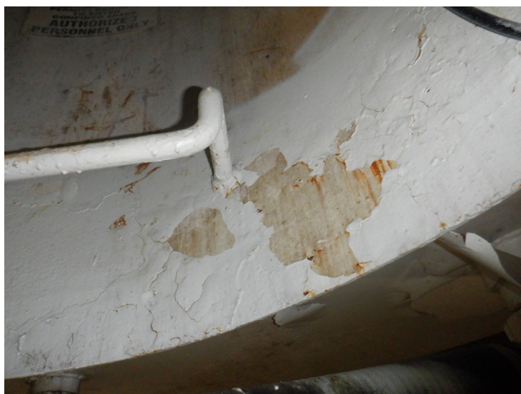
60) There are a few coating failures in the access tube.
