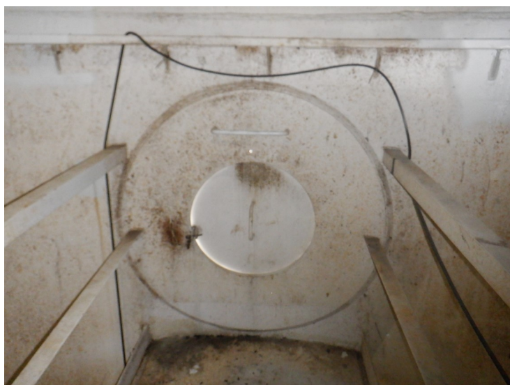
54) There is a handhold above the painter's hatch at the top of the riser.
