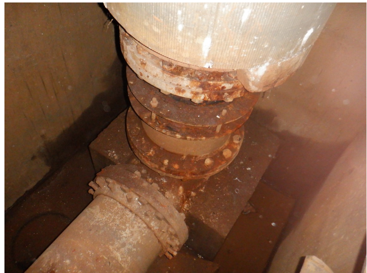
80) There is heavy corrosion on the glandular expansion joint.
