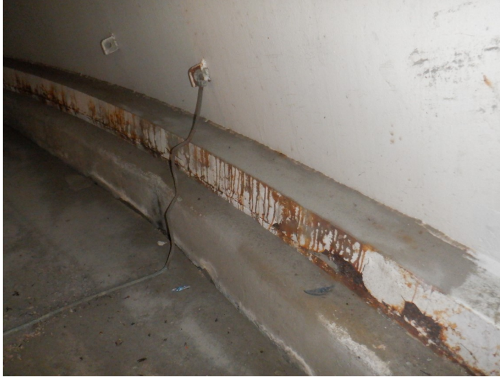
34) There are coating failures on the baseplate in the dry interior.
