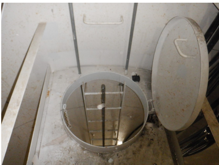
51) The ladder opening at the top platform is equipped with a hinged cover.
