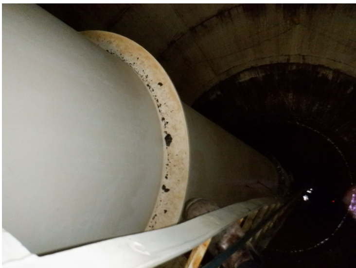
72) There are a few coating failures on the access tube above the high-water level.
