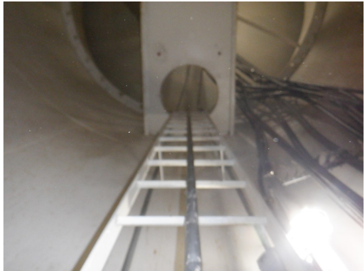
50) The riser ladder is in good condition. The ladder is equipped with a fall prevention device.
