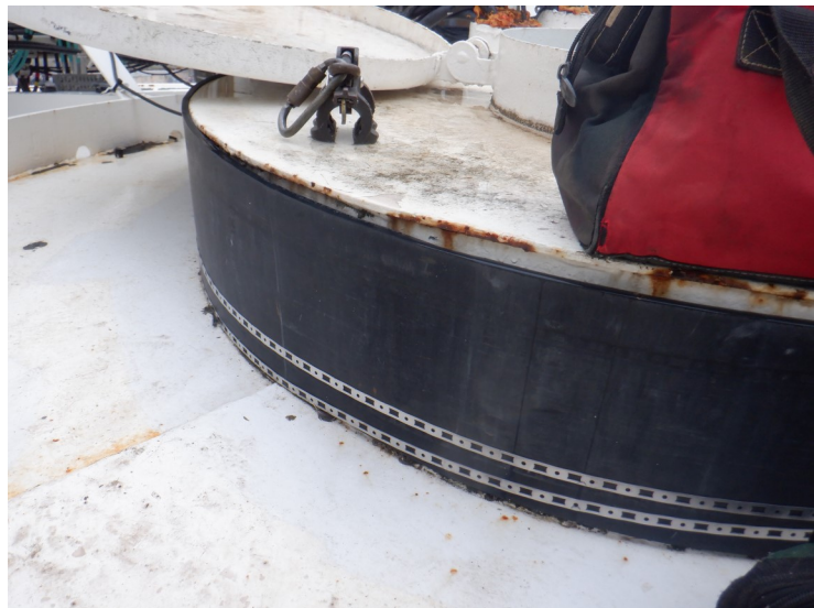
29) The access tube air gap is sealed with neoprene sheeting. One of the band clamps has slid out of position.
