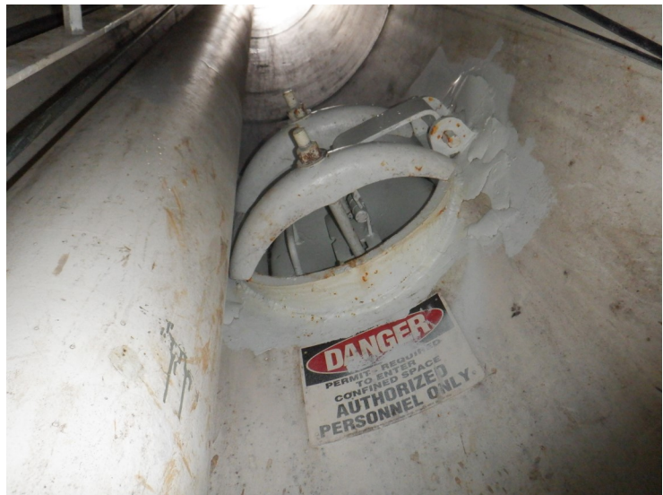
59) The manway to the wet interior in the access tube is in good condition.
