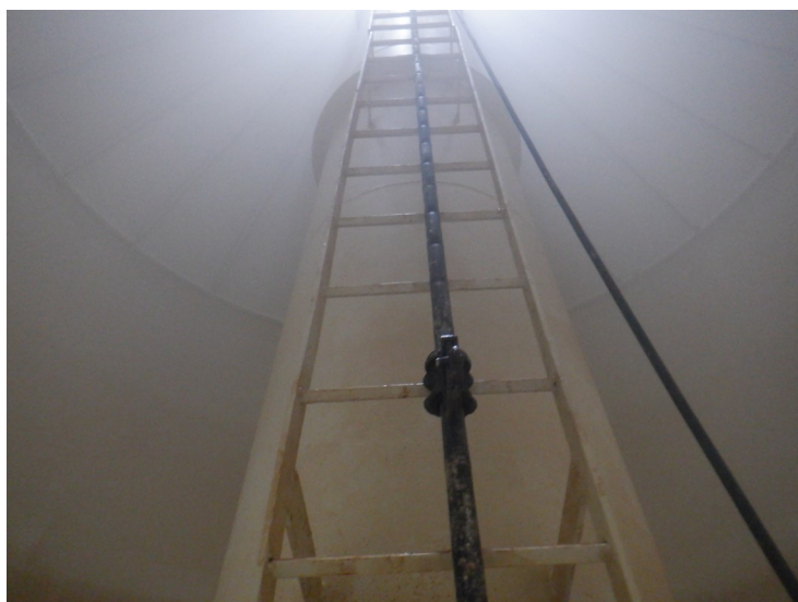
75) The wet interior ladder is in good condition. The ladder is equipped with a fall prevention device.
