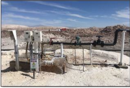
a) Brine production wells with surface equipment
