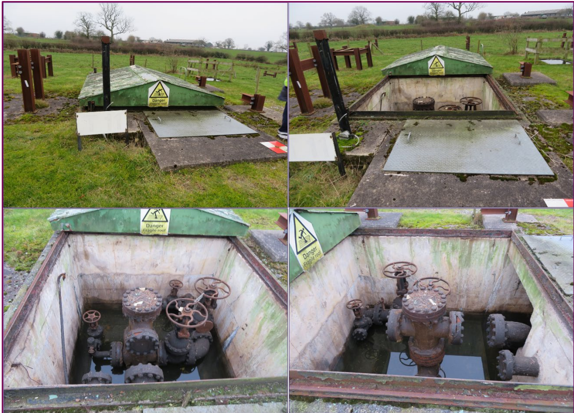
Photograph 1. Storage Cavern T11 on the Plumley PSD
