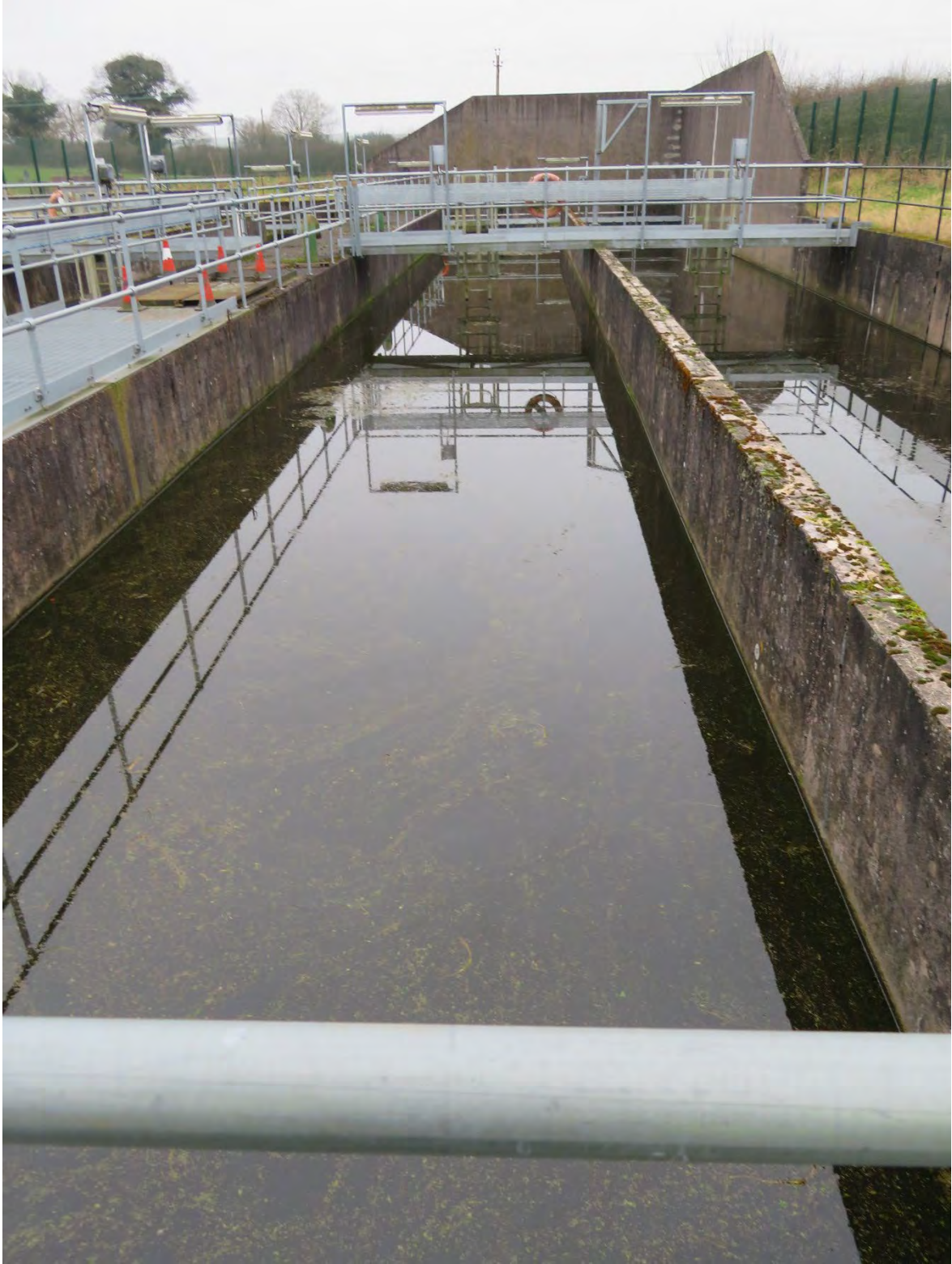
Plumley PSD Interceptor Chambers.
