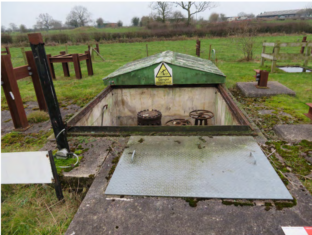
Cavern T11. Wellhead containment chamber
