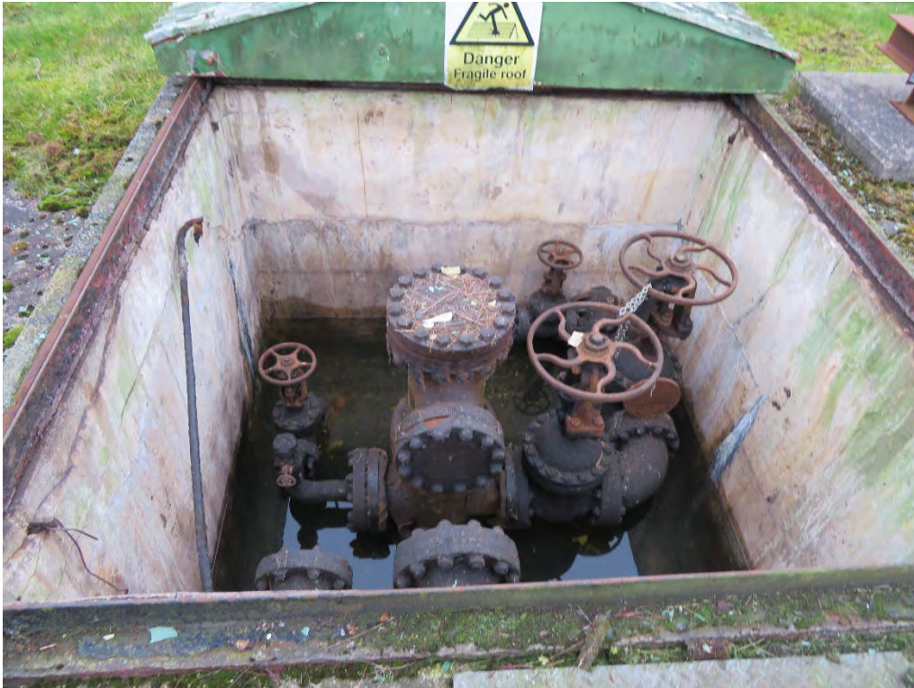
Cavern T11. Standing water in wellhead containment chamber
