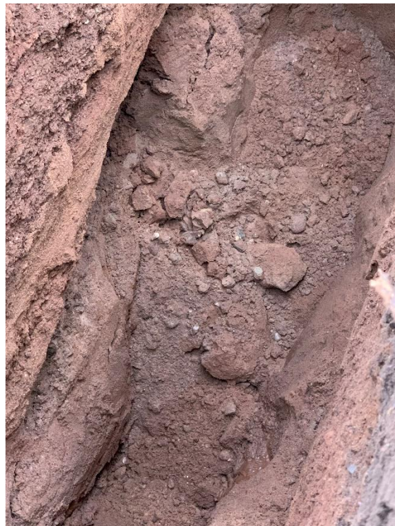
Photograph 4 – location S2B, sidewall collapse
