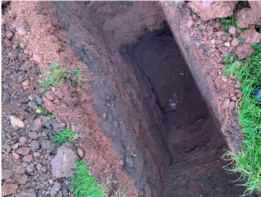
Photograph 1 - location S2, evidence of seepage at base of excavation
