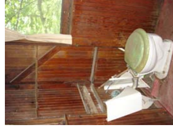
Current wall conditions in bath and kitchen; to be tiled and insulated
