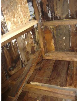
Mold and rot in north bedroom
