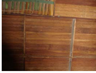
Interior walls of 1st floor bedrooms and living room; to be insulated with second layer of beadboard applied to interior
