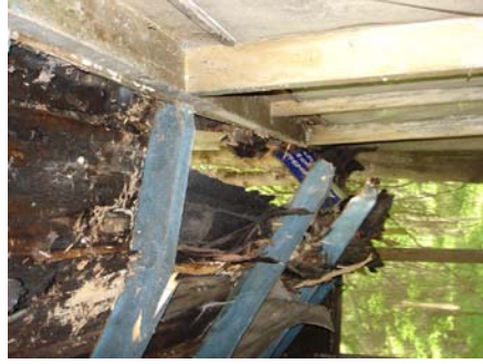
Porch roof has caved in
