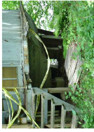
Unsound CMU foundation
