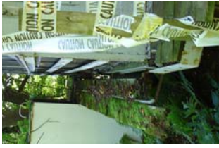
Rot on north side
