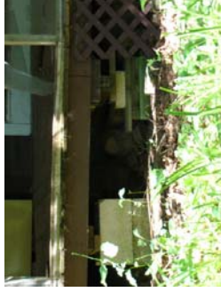
Inadequate foundation support
