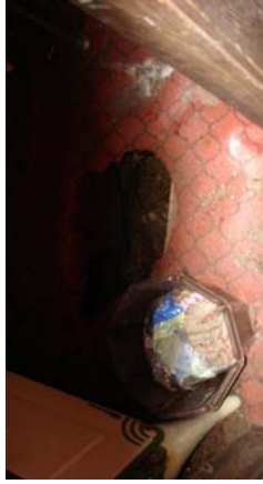
Hole in kitchen floor
