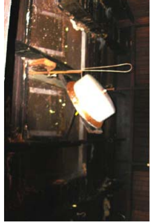
Hole in kitchen ceiling
