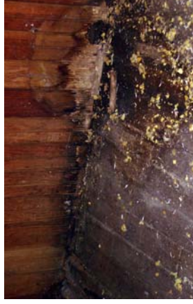
Rot along floor in west bedroom
