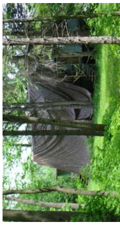
Tarp covers leaks in roof
