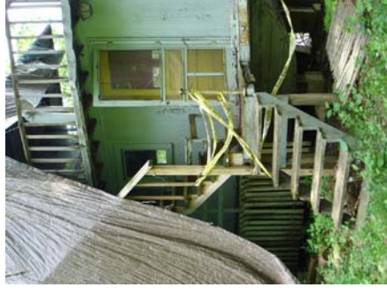
Stairs to be repaired
