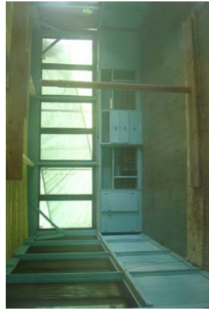
Temporary support pole in top bedroom
