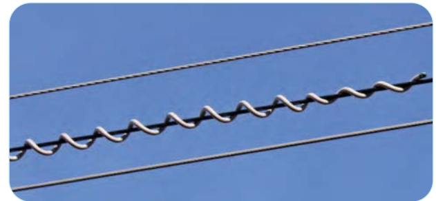
Spiral Vibration Damper on ADSS Cable
