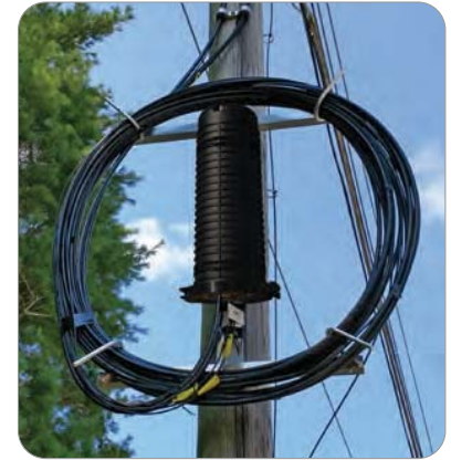
Coil Bracket holds excess ADSS cable
