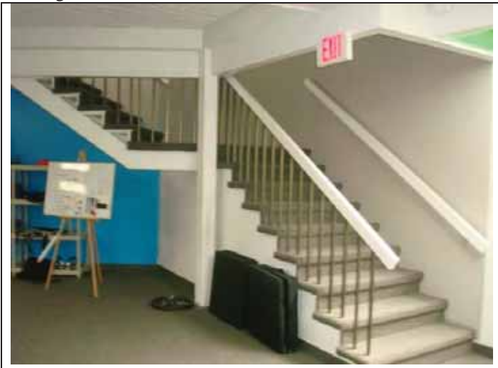
17. View of another stairwell in the Forest Fitness tenant suite in the basement of the building
