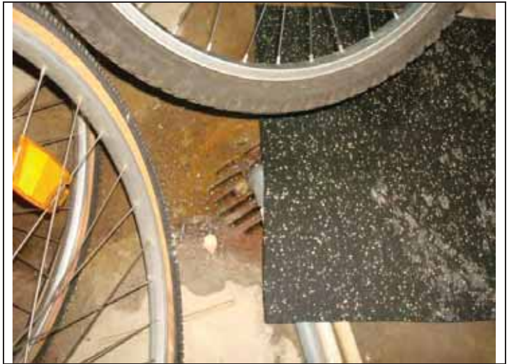
14. View of a floor drain located in the furnace room in the basement of the building
