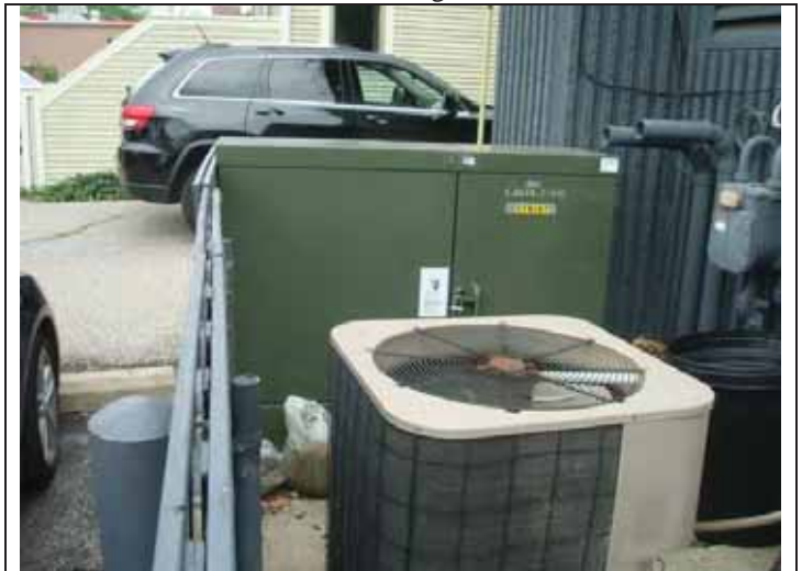
18. View of a pad-mounted transformer located near the southwest corner of the building
