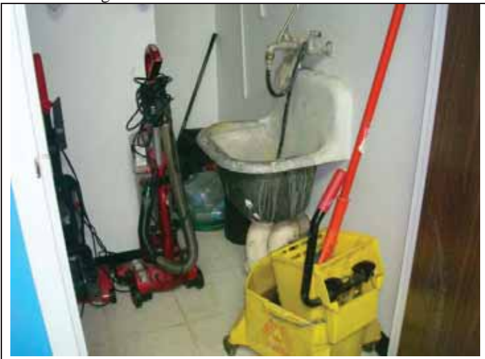
15. View of a utility room located in the basement of the building
