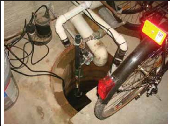
13. View of a sump located in the furnace room in the basement of the building
