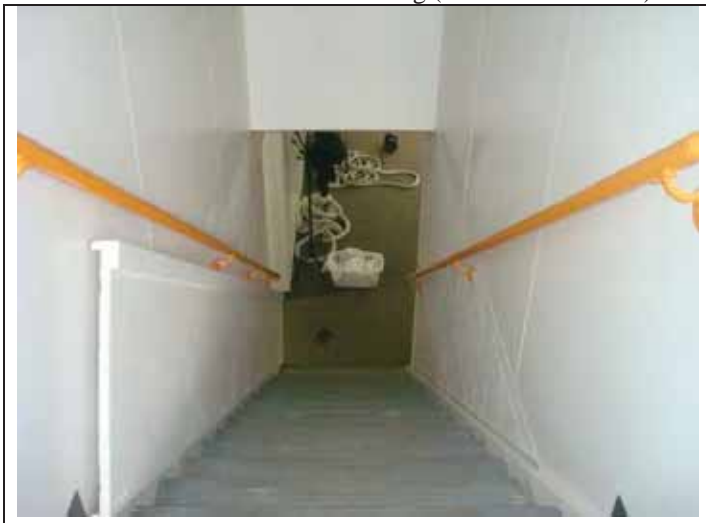
9. View of one of the stairwells to the basement tenant suite (Forest Fitness at 750 Forest Avenue)
