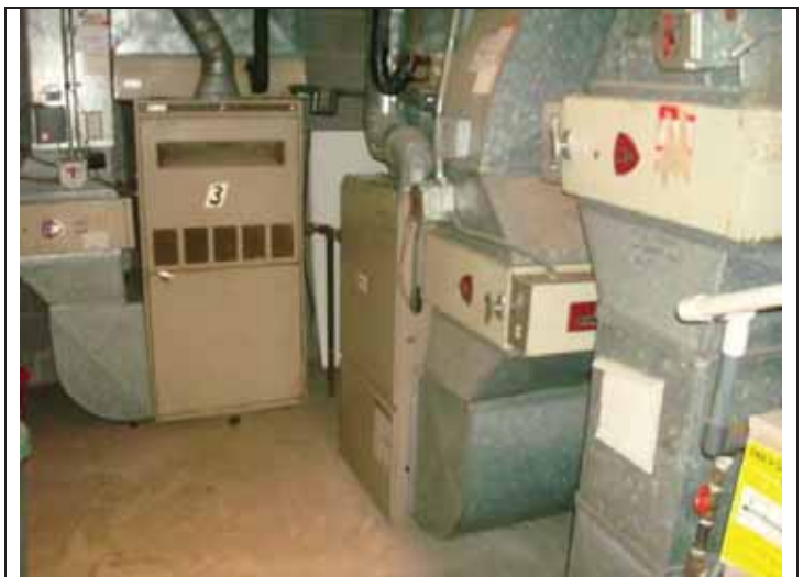
8. View of the furnace room on the first floor of the building
