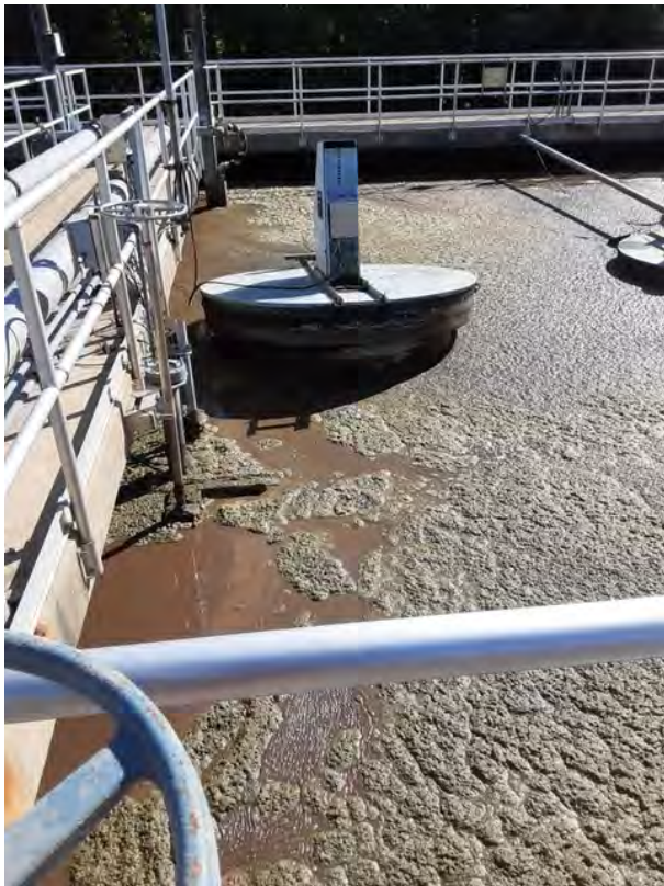
Floating decant weir
