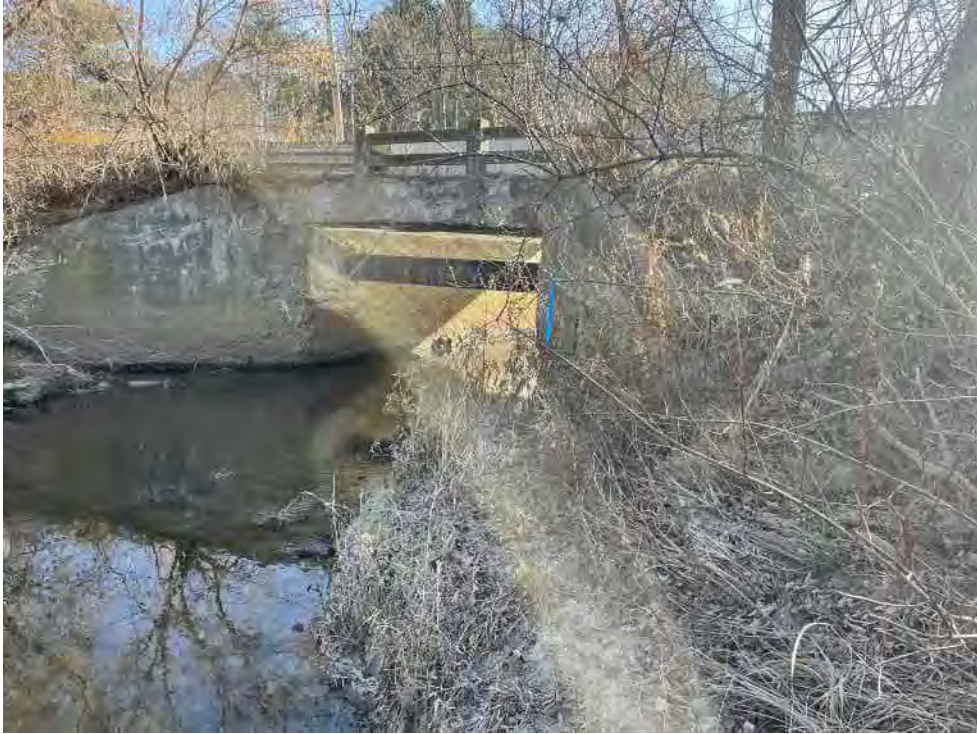
View of the B1-100 Series Bank north of the Rosemont Street Bridge—facing southeast.
