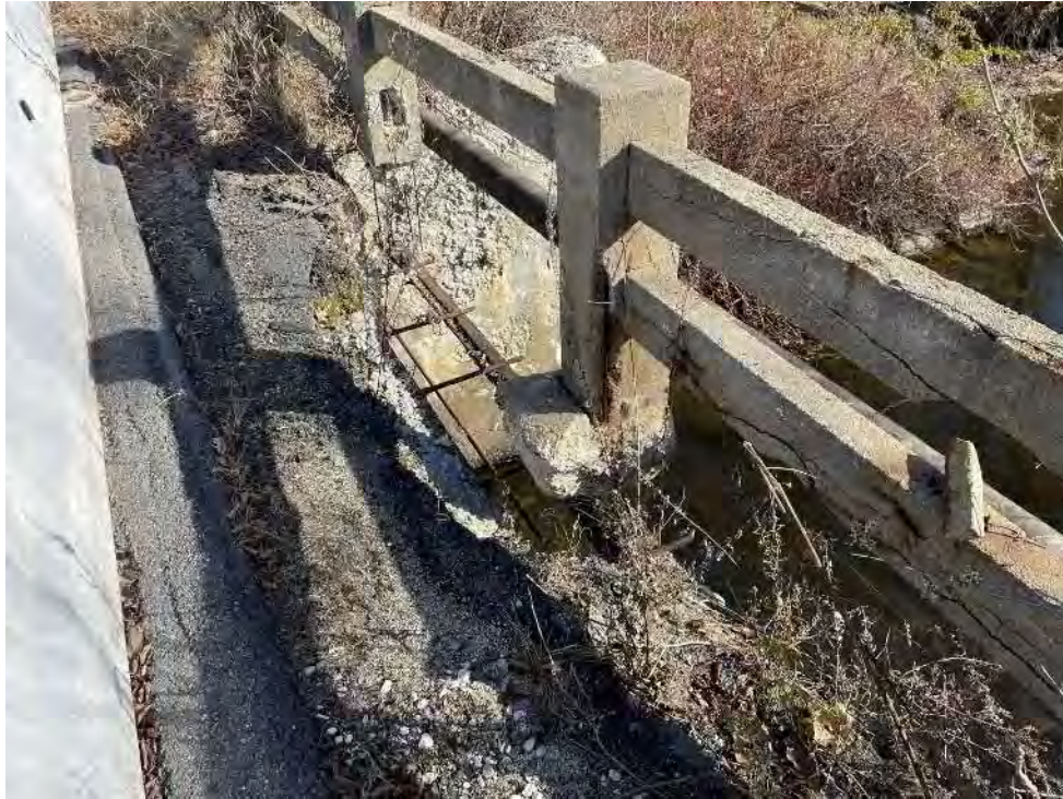
View of the current conditions of the deteriorating pavement and guard rail on the northern side of the Rosemont Street Bridge.
