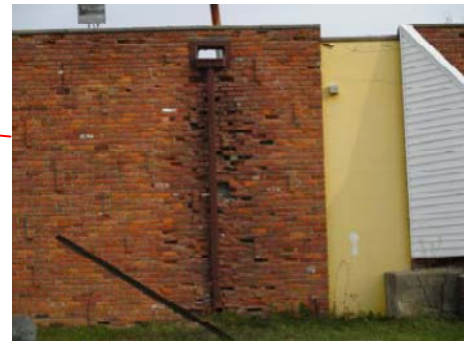
Deteriorating Building Facade
