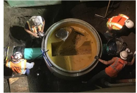
Installing a new sewer manhole as part of the wastewater replacement on Golf Club Rd
