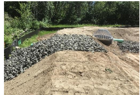
Construction of new flow control structure and emergency overflow spillway as part of modifying the existing detention storm pond at Hawks Prairie Reservoir
