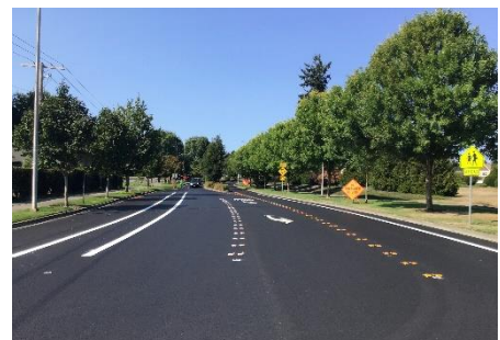
Newly installed road striping with raised pavement markers and thermoplastic lane lines along Rainier Rd in 2023
