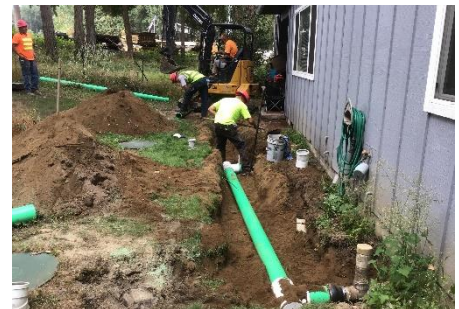
New sewer lateral installation and house infrastructure reconnection at Capitol City Golf Course
