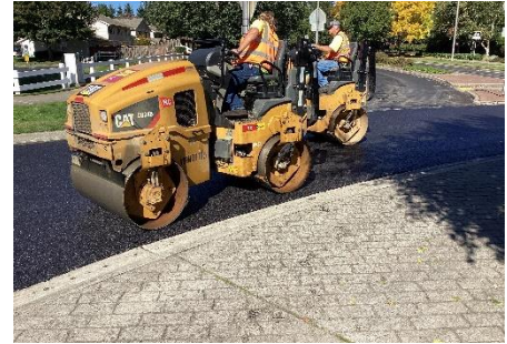
Compacting/rolling the newly laid asphalt in the roundabout at Rainier Rd and Balustrade Blvd in 2023
