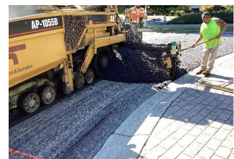
Laying asphalt in the roundabout at Rainier Rd and Balustrade Blvd in 2023
