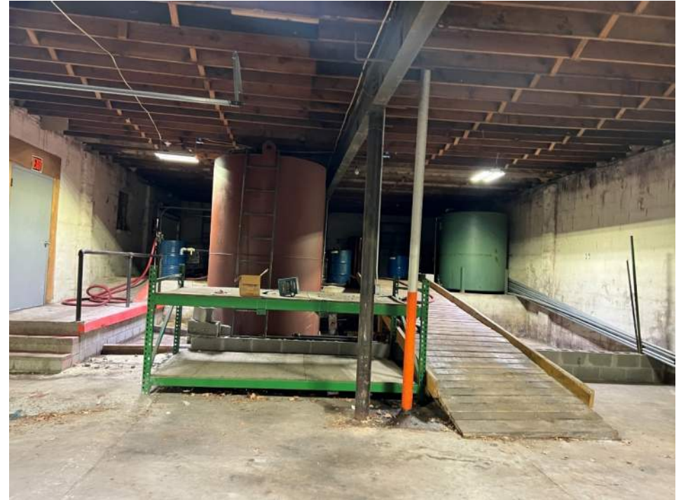
Fuel and hydraulic fluid storage inside Building C
