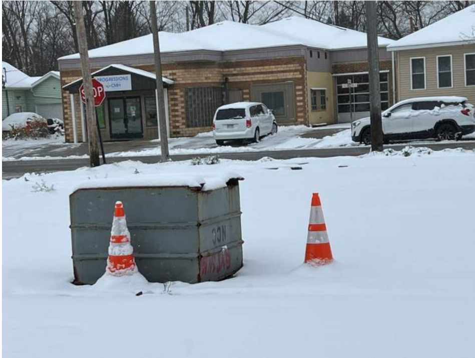
Electrical box near southwest corner of Subject Property
