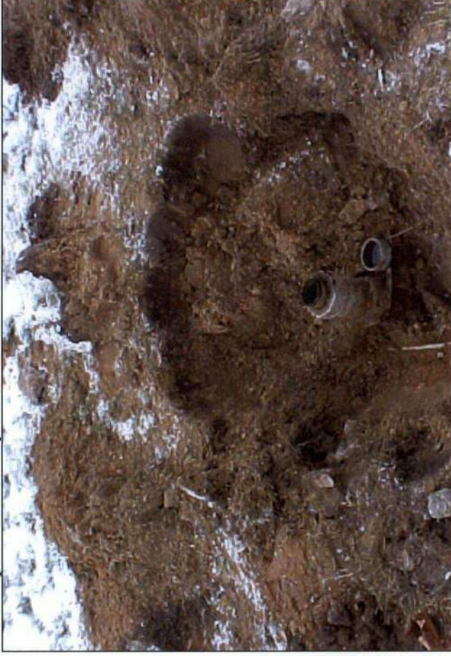
View of the fill port to the fuel oil UST. The tank was empty.
