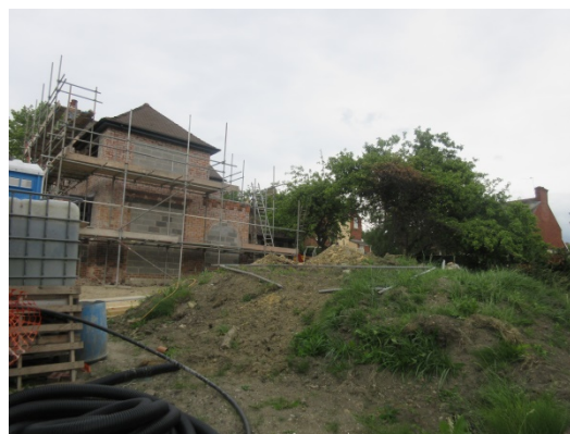
Photo taken facing north east towards the side elevation of No 12 Cavendish Street North
