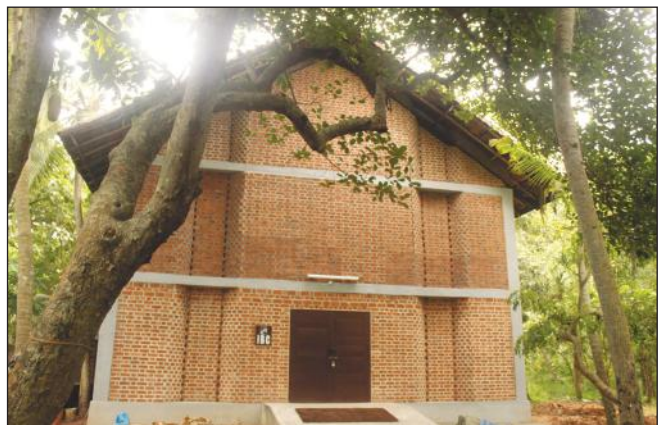
Work on the Indoor Badminton Court (IBC) with a seating capacity for 100 spectators was started during the year.
