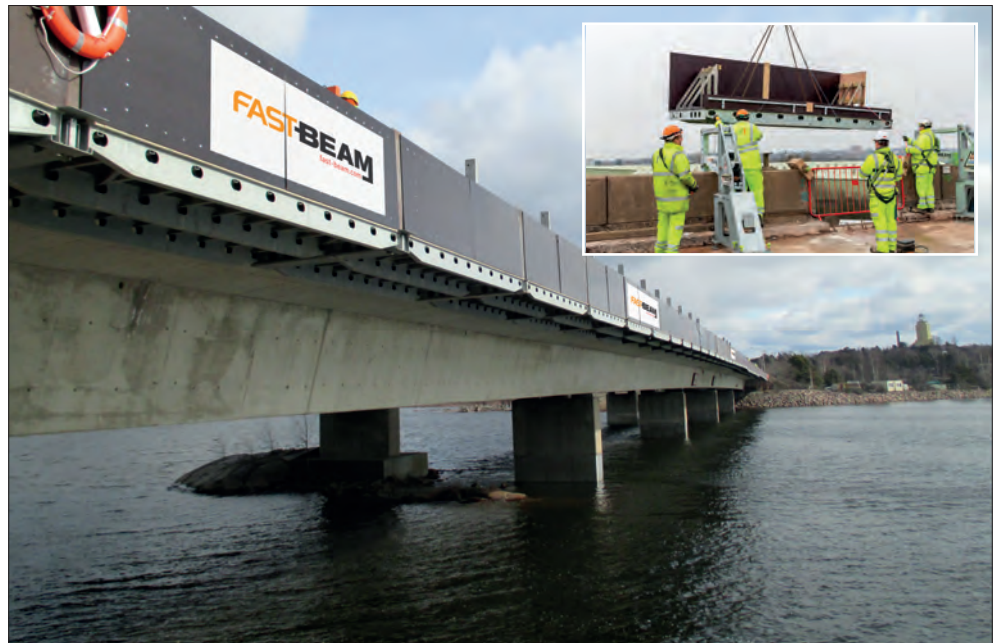
Main picture: Fast Beam access technology Inset: VolkerLaser conducting the trial on the M5 Oldbury Viaduct
