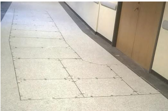
PS4300 Special recessed tray type, this cover was installed at Llandough Hospital in Cardiff. This unit featured a number of obscure angles and was over 8m in length.
