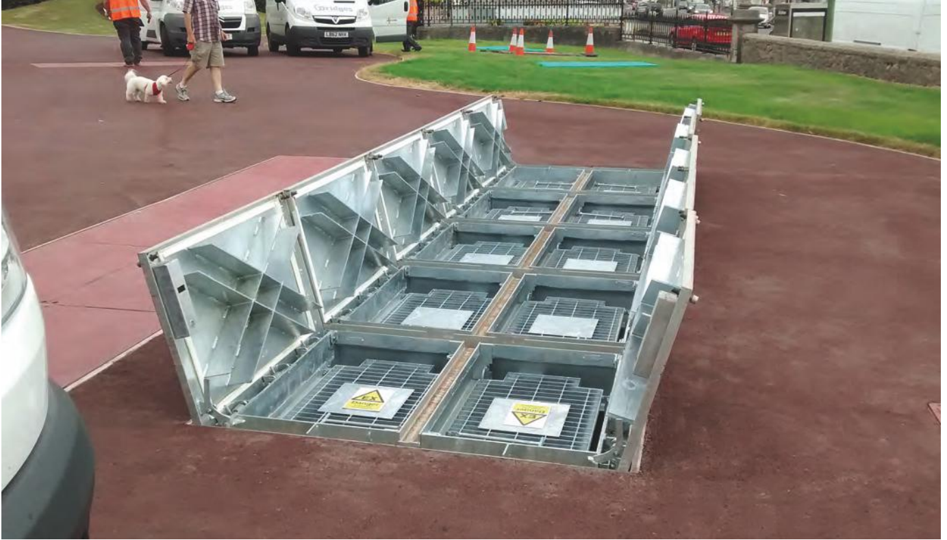
PS1680 5x2 Configuration multiple spring assisted cover and frame installed at Abbey Gardens on the south coast. Due to the location of these covers they required red anti slip coating to blend in with the surrounding area.
