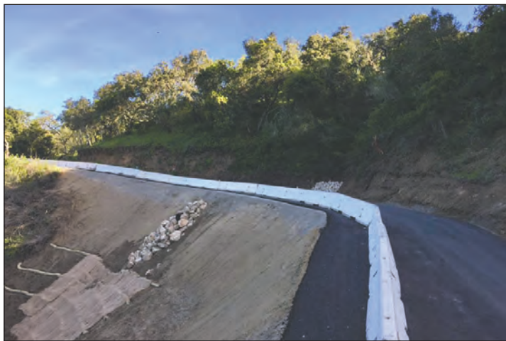
A one-lane temporary road was opened on Cachagua Grade last spring so locals could use the road, but now it's closed again while Granite Construction works on a permanent fix.
