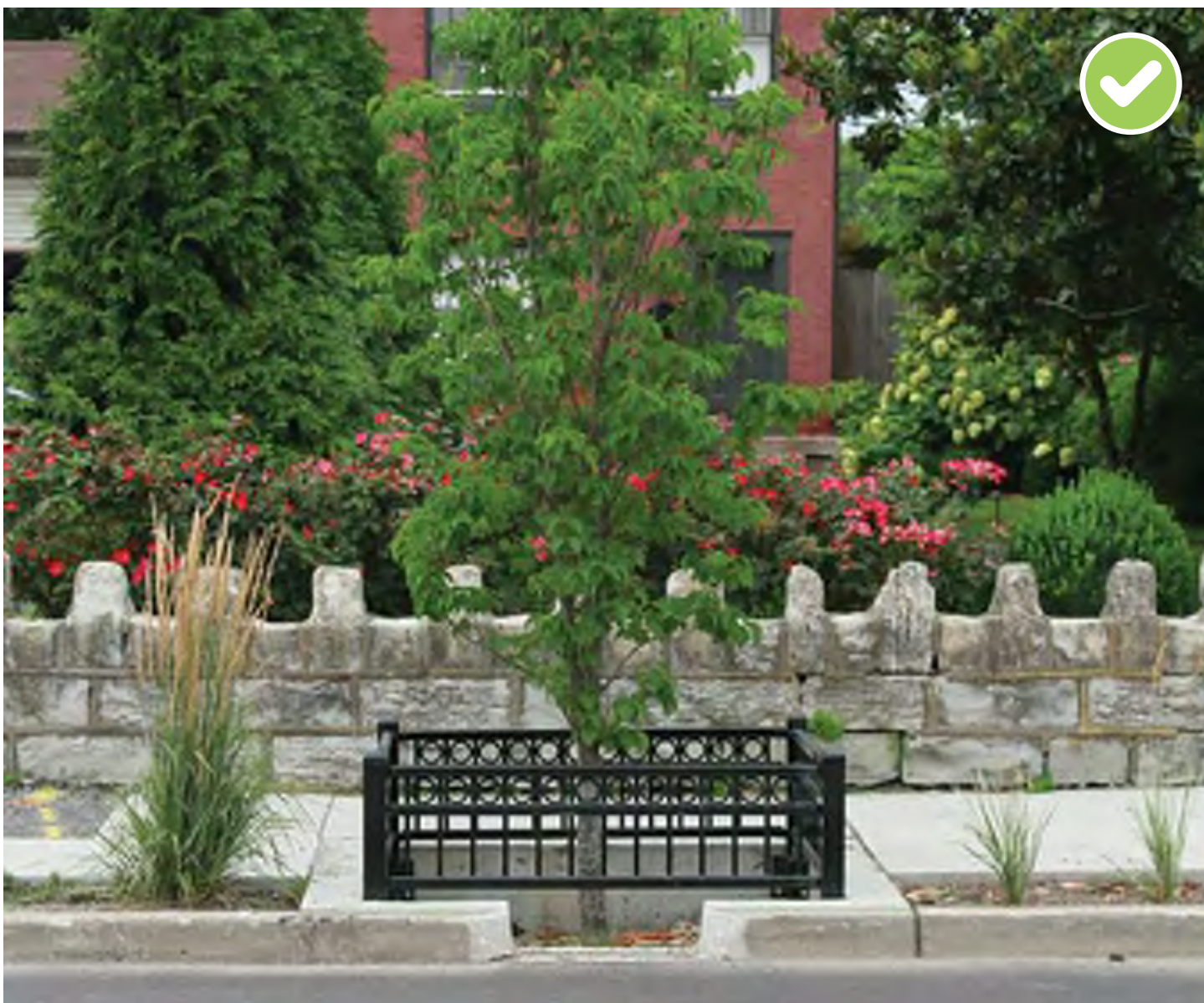
This stormwater tree pit demonstrates a structurally and functionally sound stormwater feature.
