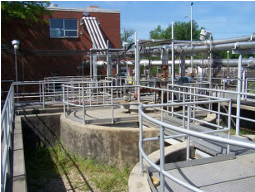
Figure 3.4-1 Photo of Vortex Grit Chamber at CRW AWTF
