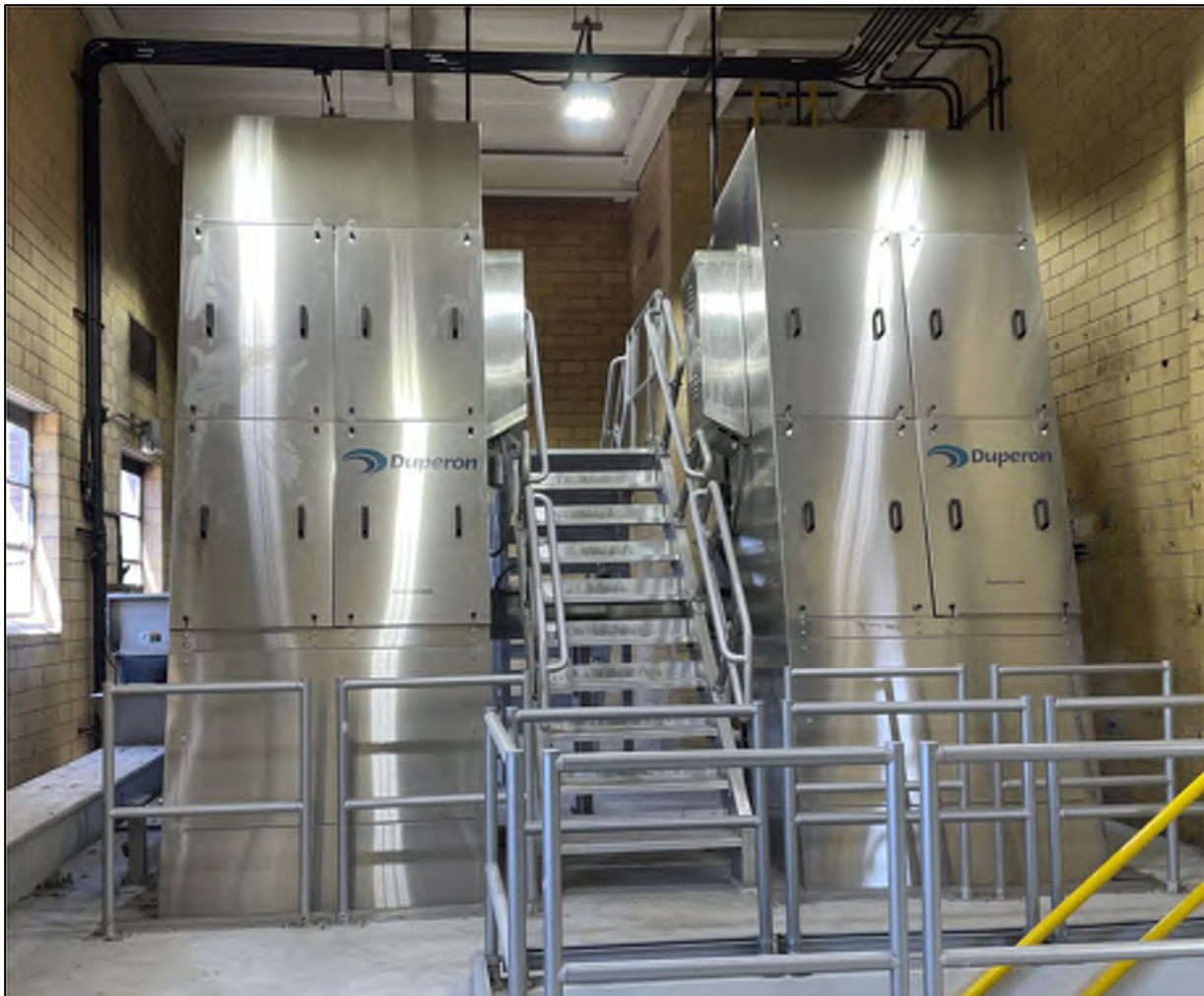
Figure 4.3-4 Front Street Pump Station Bar Screens
