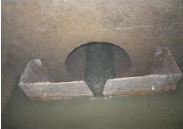
Regulating Chamber Effluent
