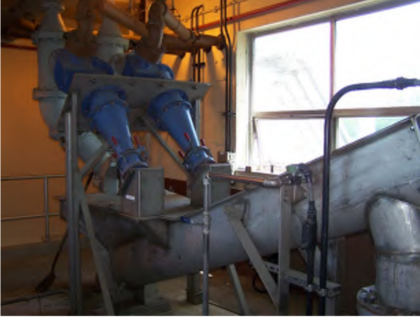
Figure 3.3-2 Photo of Classifier Unit at the CRW AWTF
