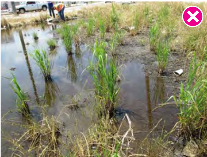
Water should drain from properly-functioning SCMs within 3 days after a rainfall; if it does not, there may be a serious problem.
