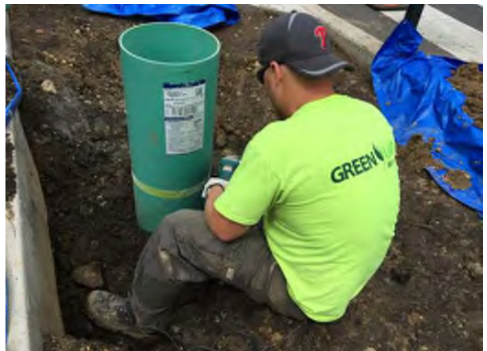
Maintenance personnel reconstructing the domed riser within a bumpout based on the redesign from the engineer.
